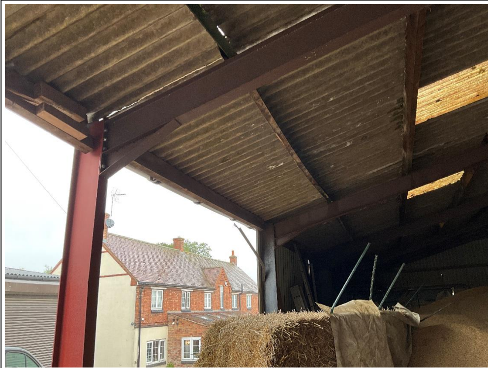
3.- Underside of roof, note purlin distortions
