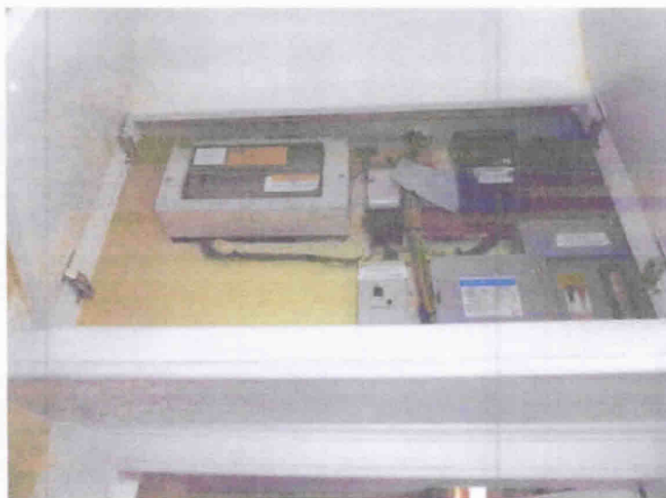
main house distribution board
