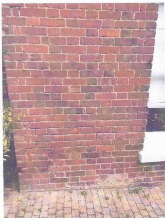
section of eroded mortar to LH side wall.
