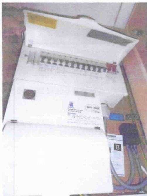
Stable flat distribution board.
