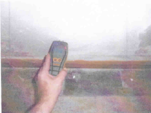
dampness to flat stairwell wall
