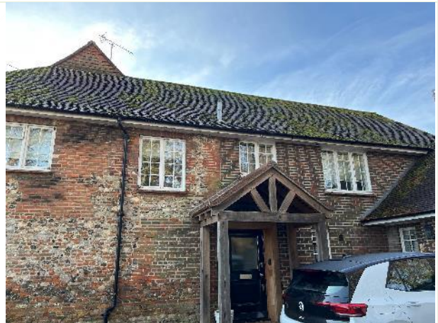
Front of the surveyed house (northern aspect) that is not affected by the proposed works.
