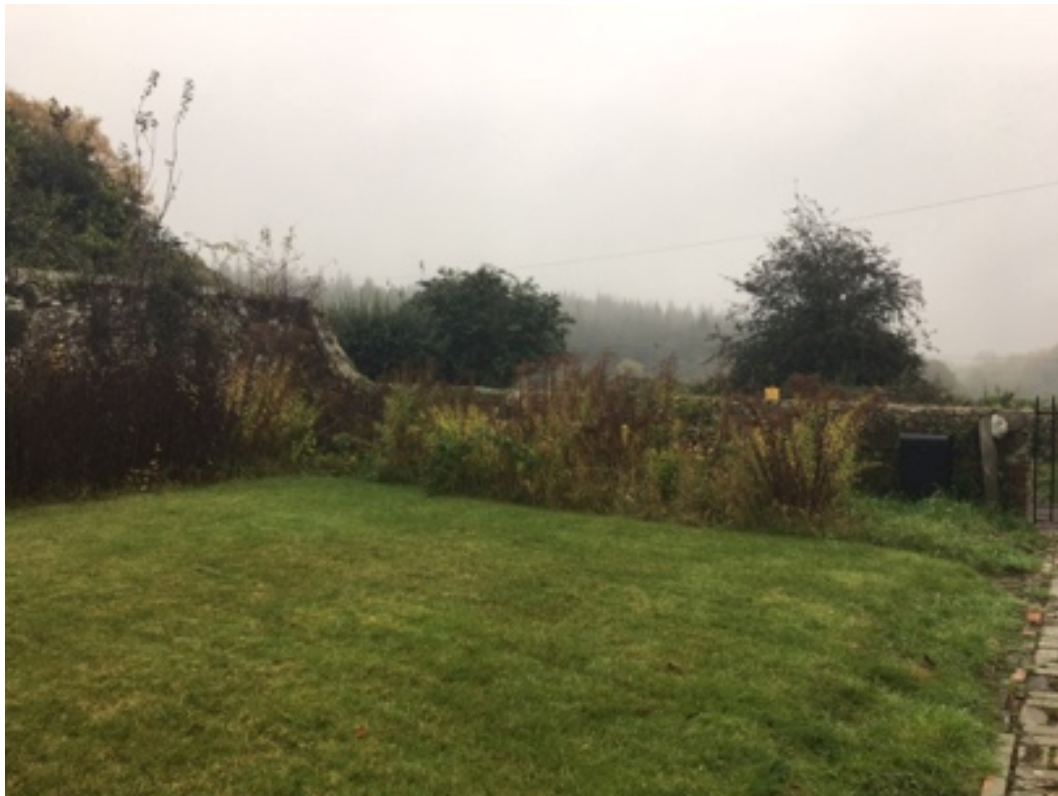
The stone boundary wall at the north-eastern corner of St Peters Well, constructed in local greensand stone
