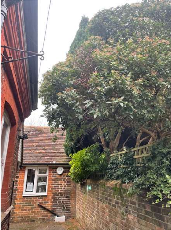
Photo 2. Showing T3 close/touching Parish Hall.
