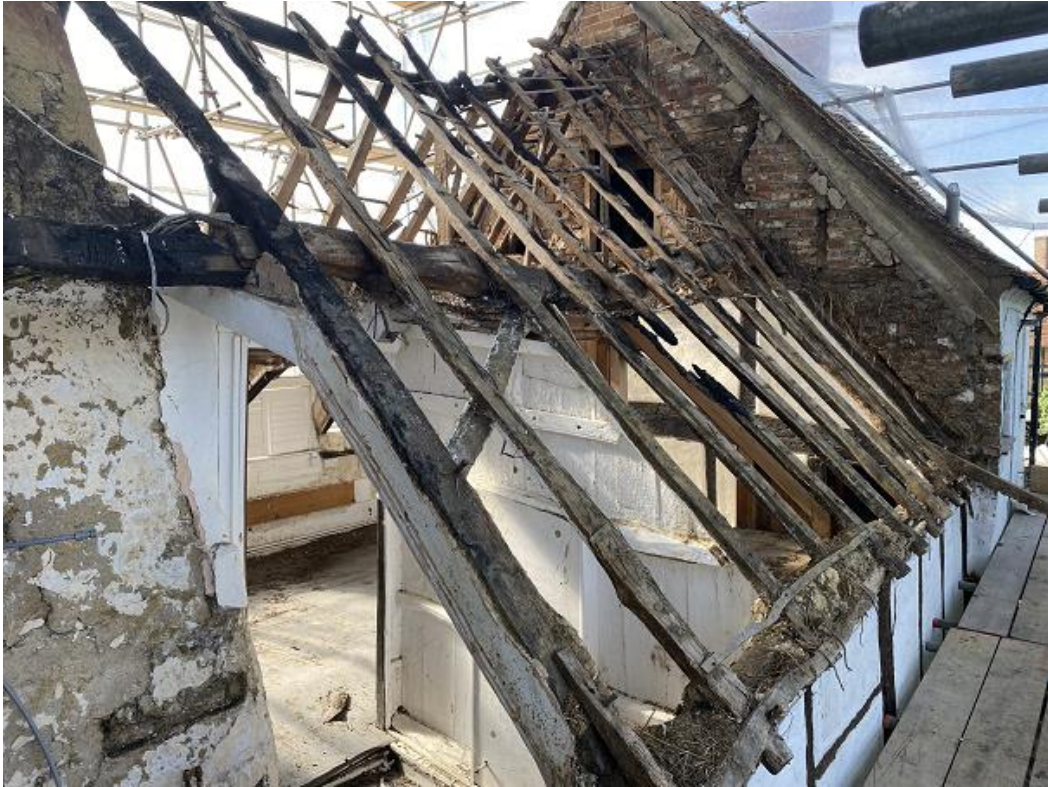
Plate 3: North-facing roof slope looking west, showing bracing timber beneath purlin and small section of riven lath to lower area
