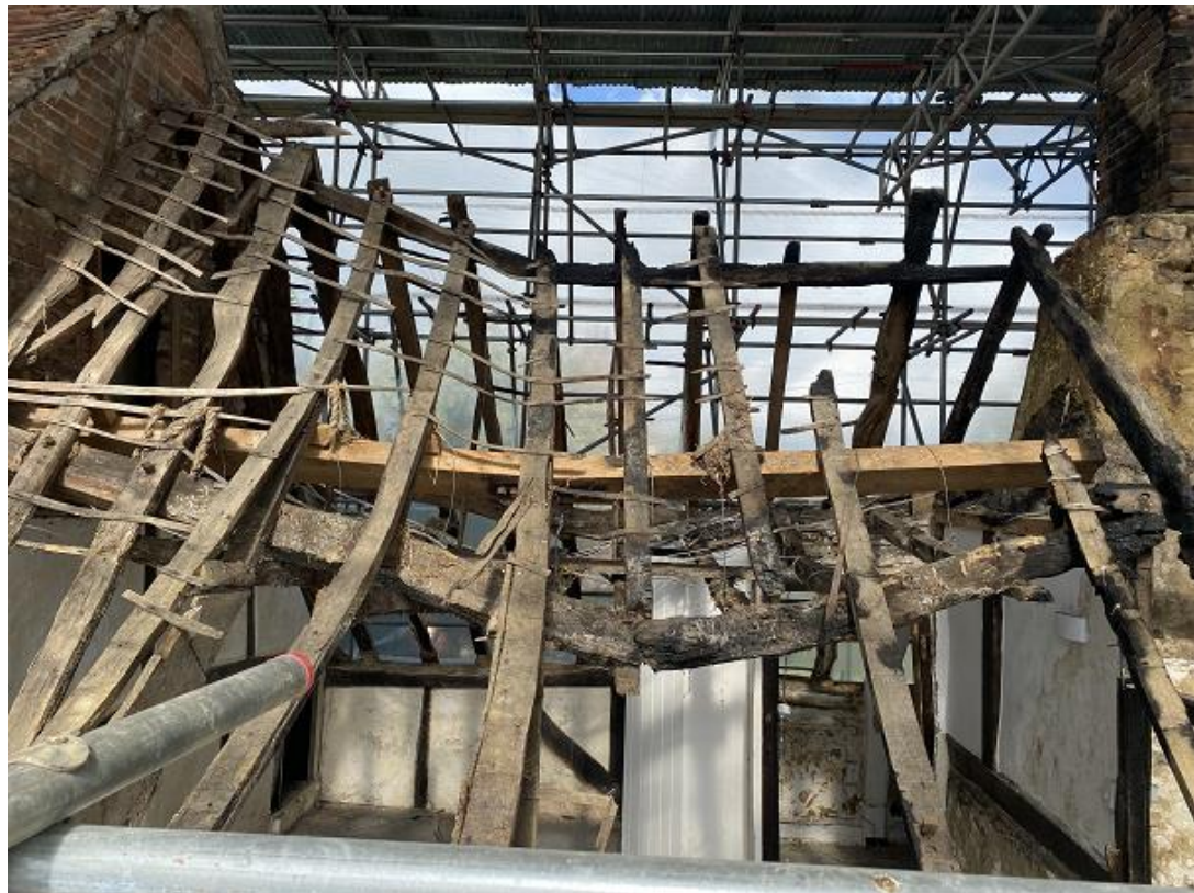
Plate 8: South-facing roof slope looking north, showing failed purlin with modern purlin over
