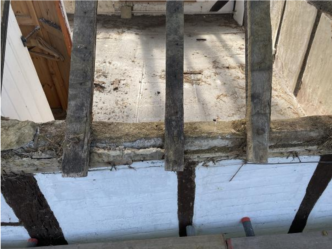
Plate 5: North-facing roof slope looking south, showing pegged connection of rafters into wall plate
