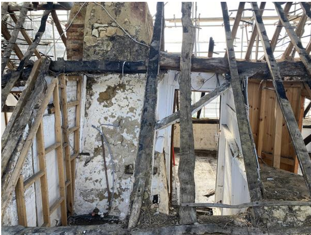
Plate 4: North-facing roof slope looking south, showing connection of brace into rafter and purlin
