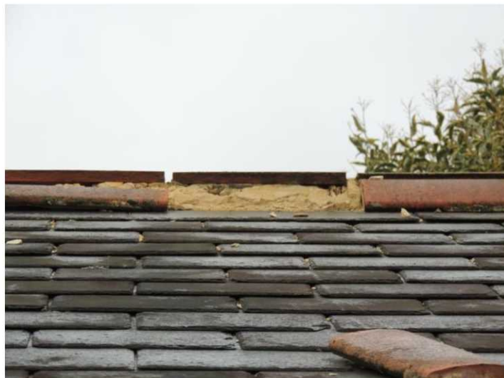
Photo 7: Cement where a ridge tile has slipped
