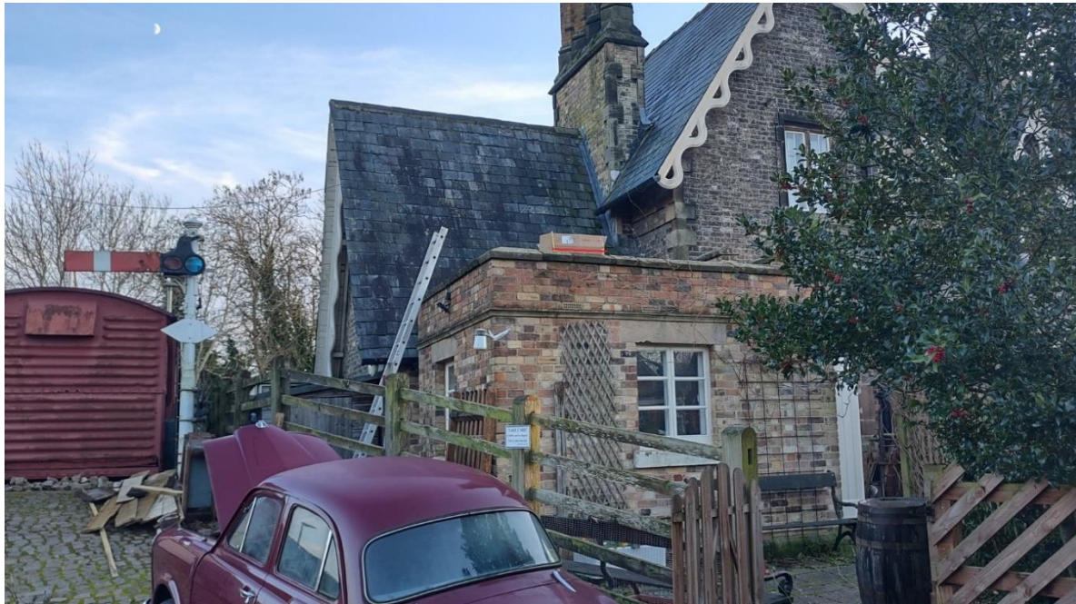
The view from street level in The Sidings. The red line is only just visible. With two more courses of brick, it will be completely hidden.
