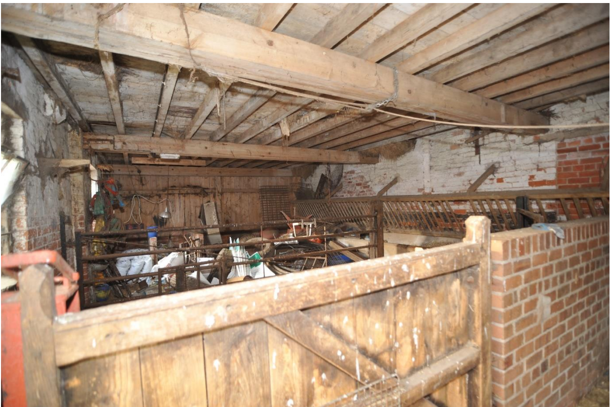
Pl.9: Interior of the central section, looking west and showing the inserted loft floor.
