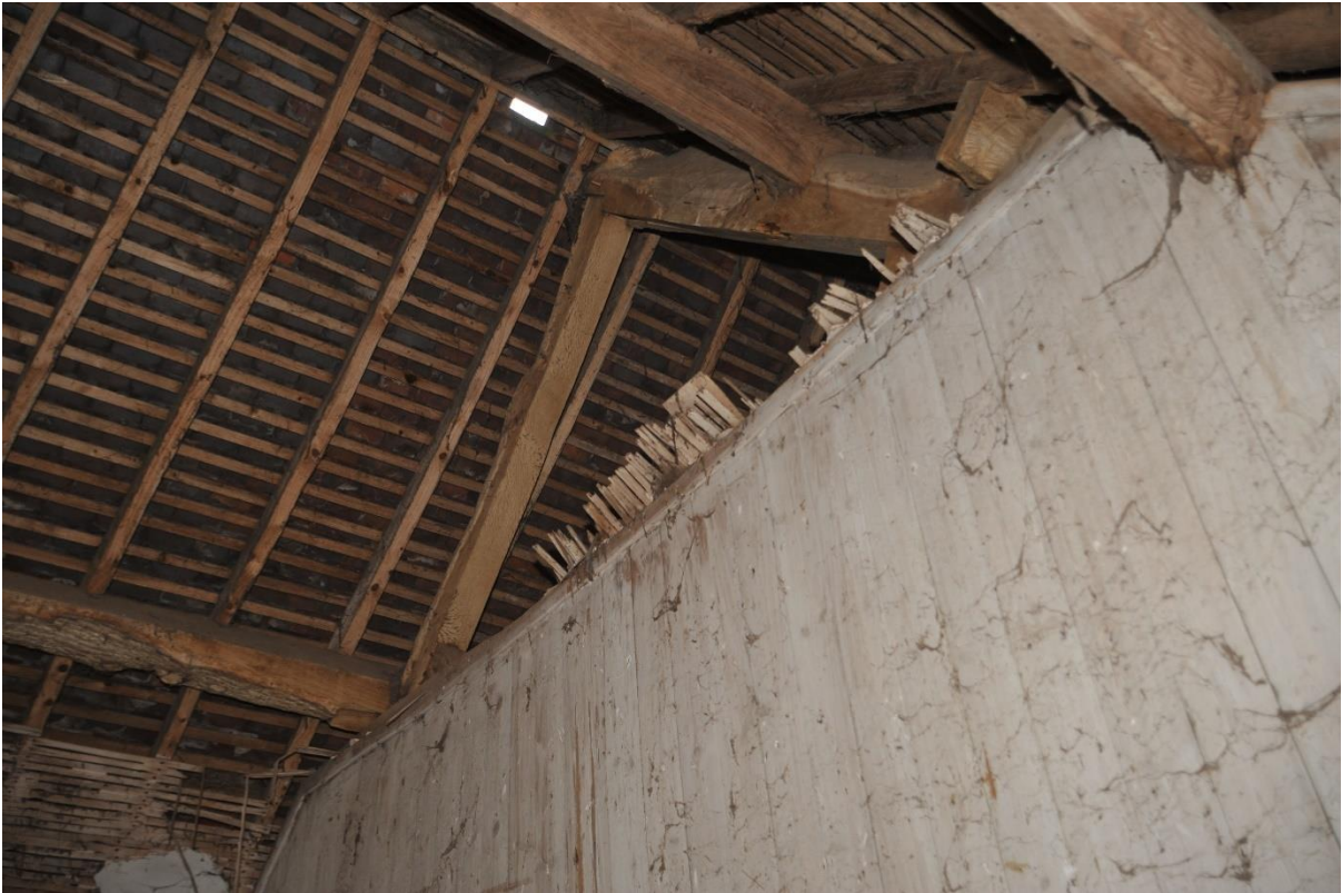
Pl.8: Part of the roof structure, showing an open truss of unknown provenance.
