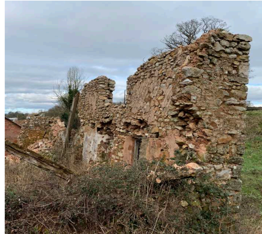
View of the north wall, showing the significant leaning and loose stones. (02/23)
