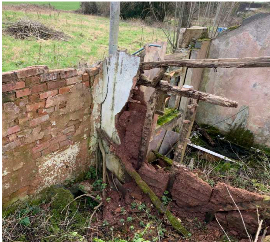
View of a section of the east wall and window from the inside, looking at the assumed former bathroom. (02/23)
