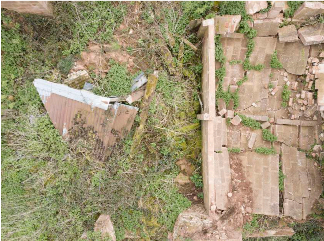
Aerial view showing details of collapsed blockwork and roof sections (04/22)
