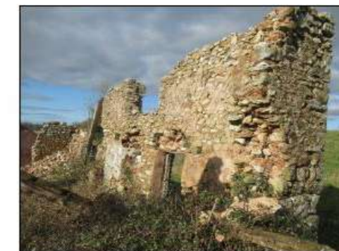
Leaning north wall.
