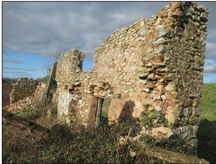
Leaning north wall.
