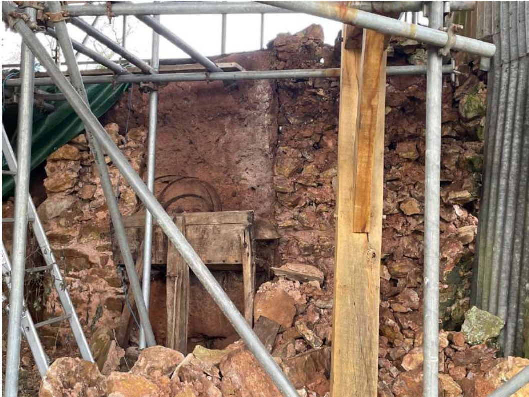
Photo 17: Crevices in Barn 1 stonework.
