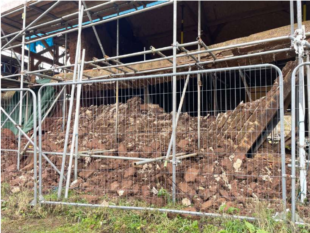
Photo 15: Collapsed west elevation of Barn 1.
