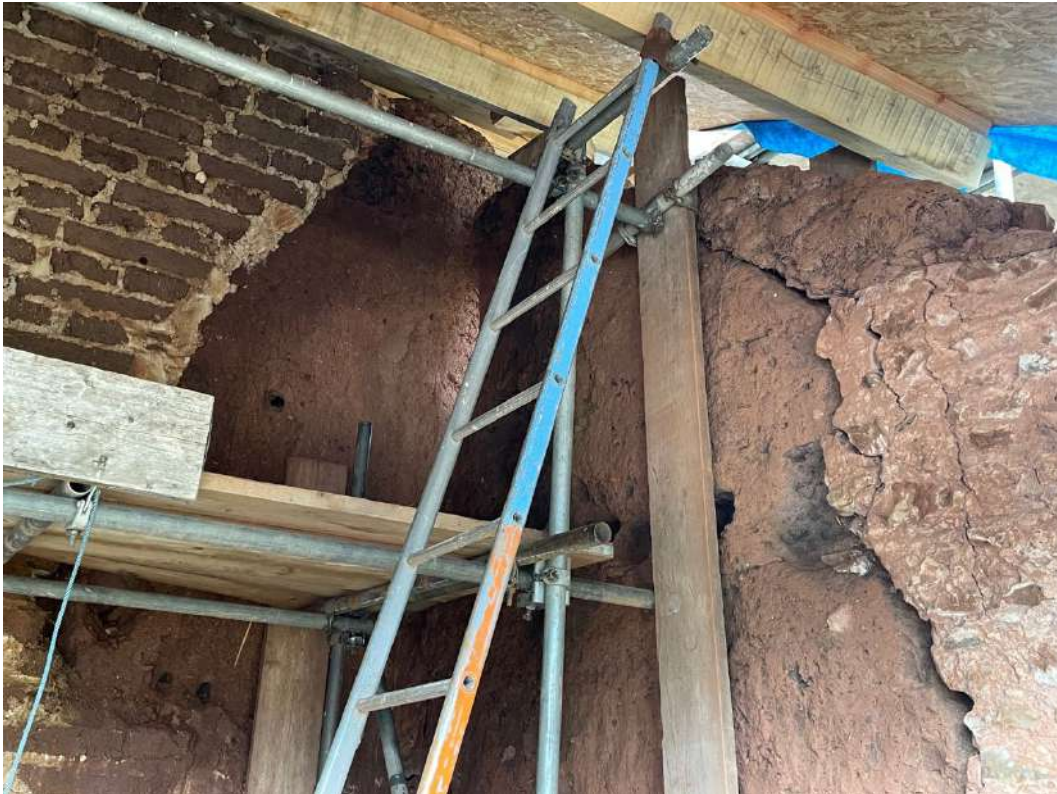
Photo 19: Crevices in Barn 1 cob.
