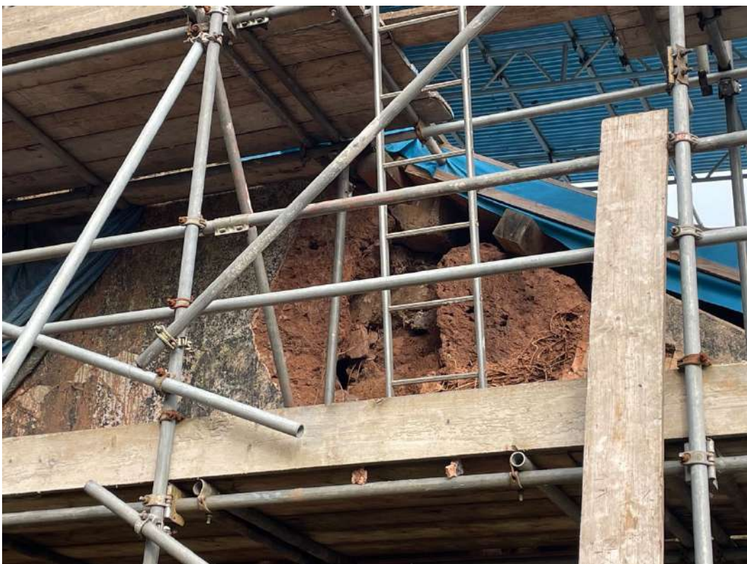
Photo 20: Crevices in Barn 1 cob.
