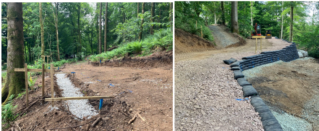
Figure 5: Images extracted from HBB website showing examples of the foundations and retaining wall.
