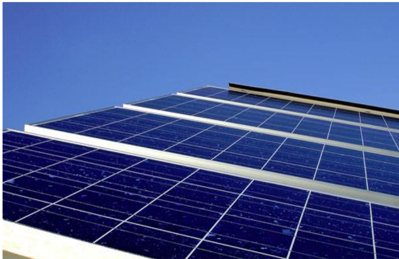
Figure 6. Typical PV Panel
