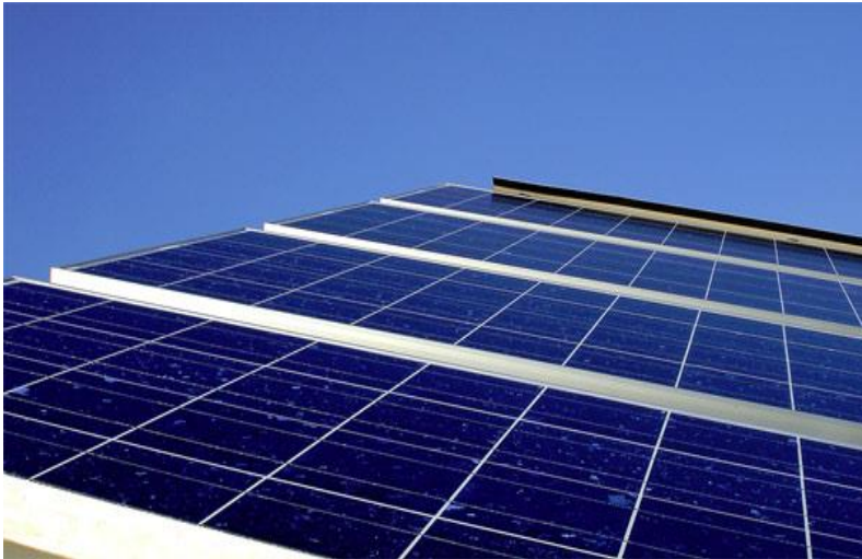
Figure 10. Typical PV Panel
