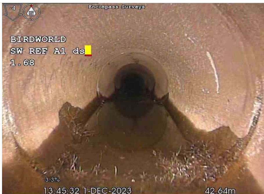
2-1-14A, 00:02:46, 42.64 m Roots, mass at joint, 10% cross-sectional area loss, start
