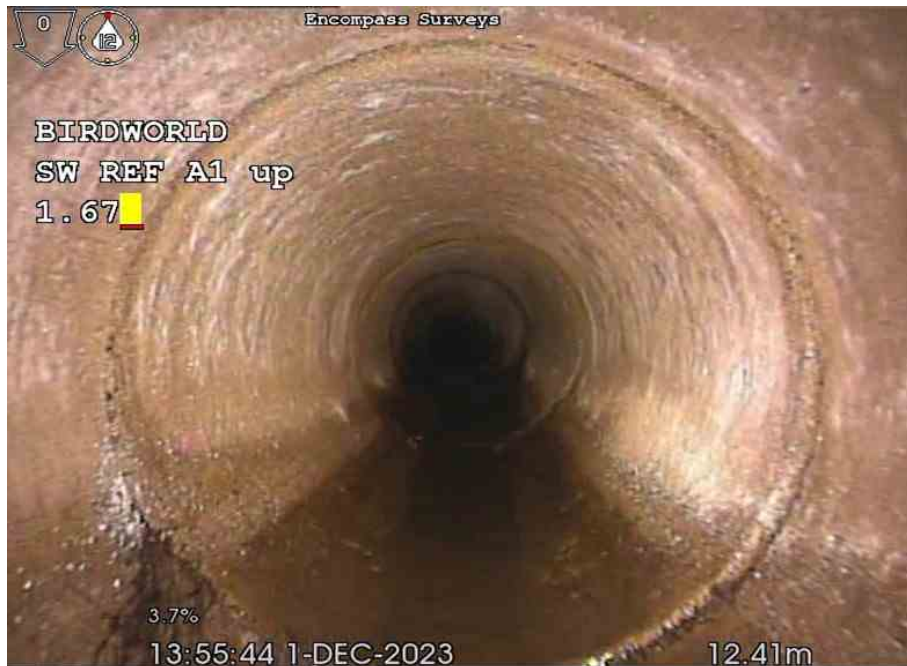
1-1-5A, 00:00:51, 12.41 m Roots, fine at joint
