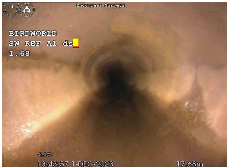
2-1-5A, 00:01:11, 17.68 m Crack, longitudinal at 9 o'clock, start
