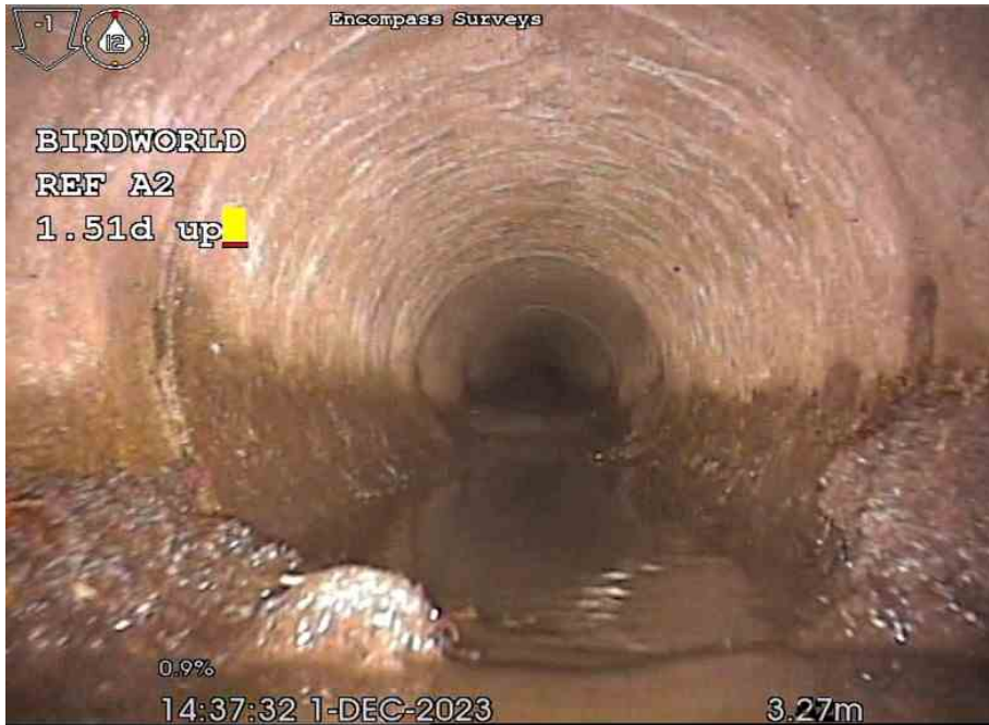
4-1-3A, 00:00:15, 3.27 m Roots, mass at joint, 10% cross-sectional area loss, start
