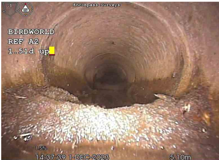
4-1-3B, 00:00:15, 3.27 m Roots, mass at joint, 10% cross-sectional area loss, start
