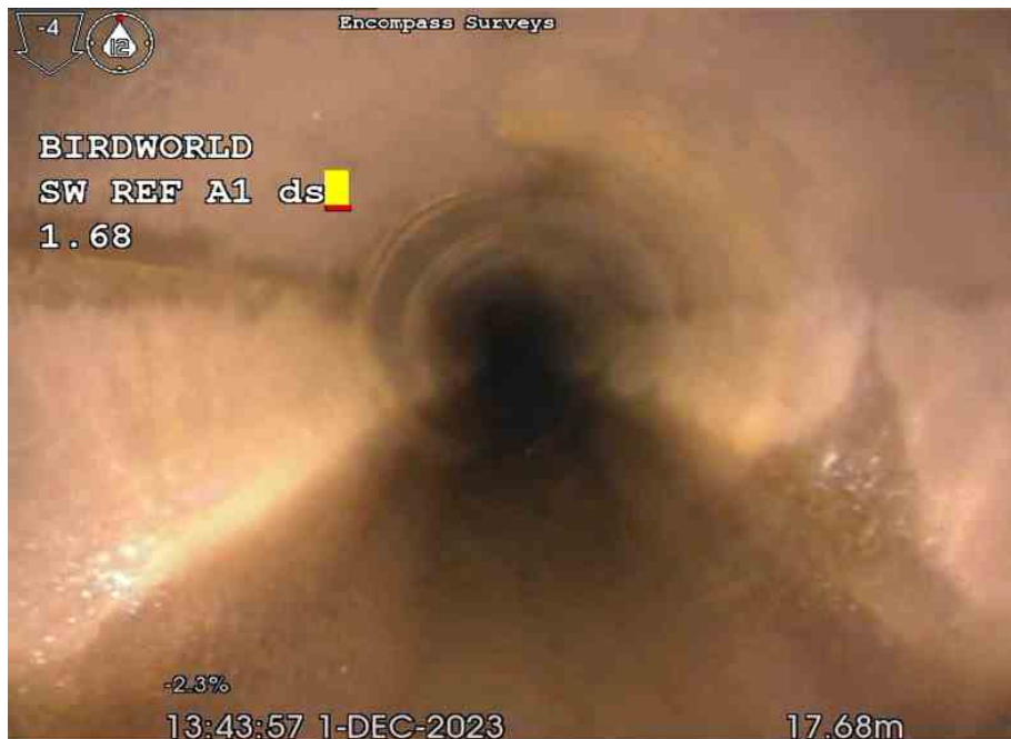
2-1-4A, 00:01:08, 16.59 m Crack, longitudinal at 2 o'clock, start
