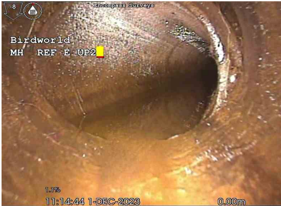
10-1-2A, 00:00:01, 0.00 m Joint displaced, large
