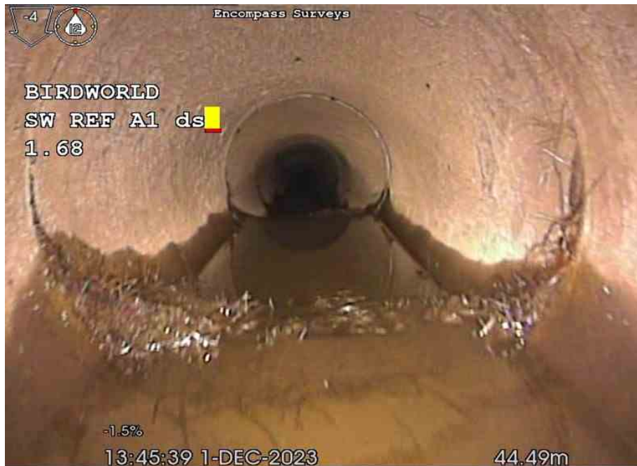
2-1-14B, 00:02:46, 42.64 m Roots, mass at joint, 10% cross-sectional area loss, start
