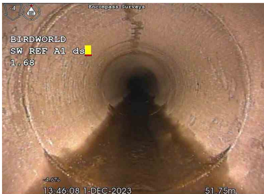
2-1-16A, 00:03:22, 51.75 m Crack, longitudinal at joint at 12 o'clock
