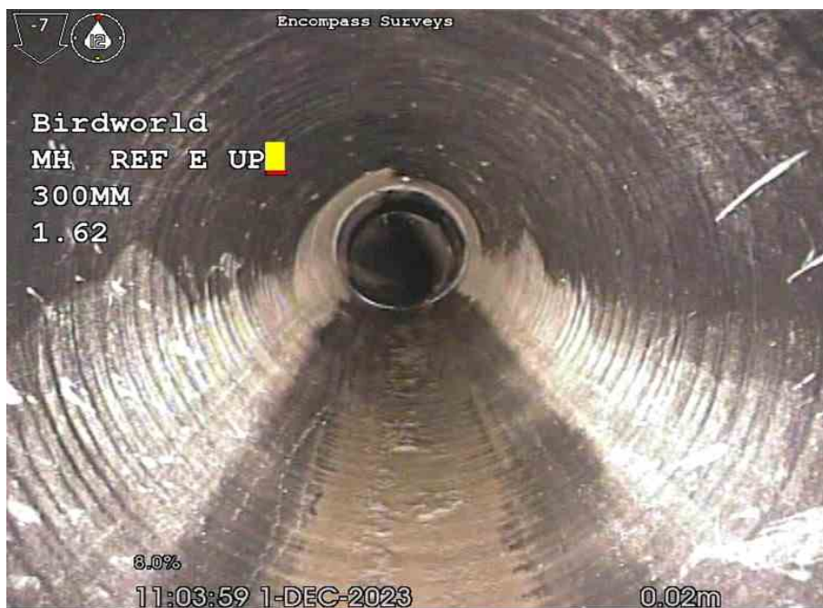
9-1-3A, 00:00:00, 0.00 m Settled deposits, fine, 5% cross-sectional area loss, start
