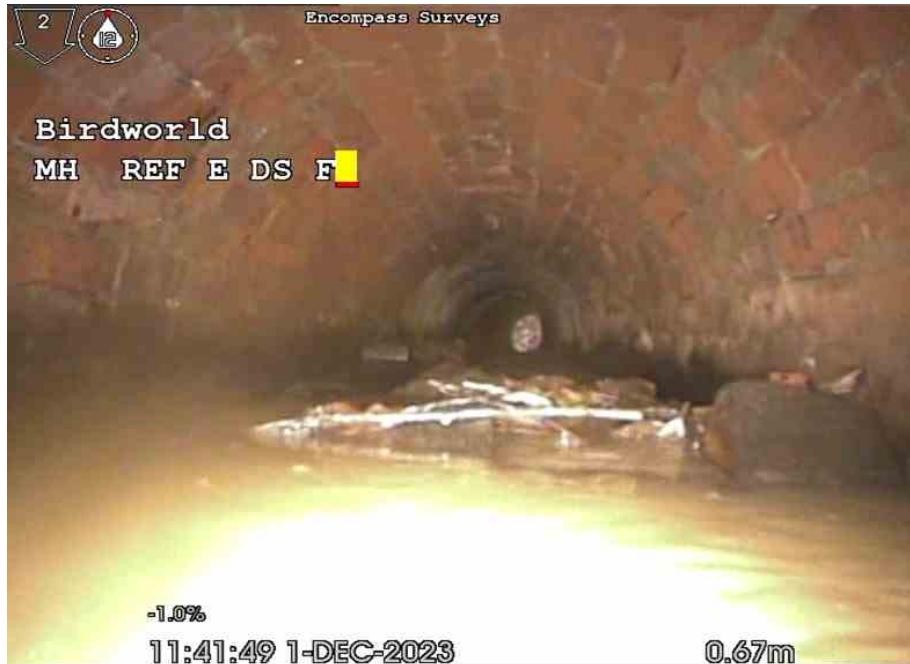
8-1-5A, 00:00:06, 0.67 m Settled deposits, coarse, 25% cross-sectional area loss
