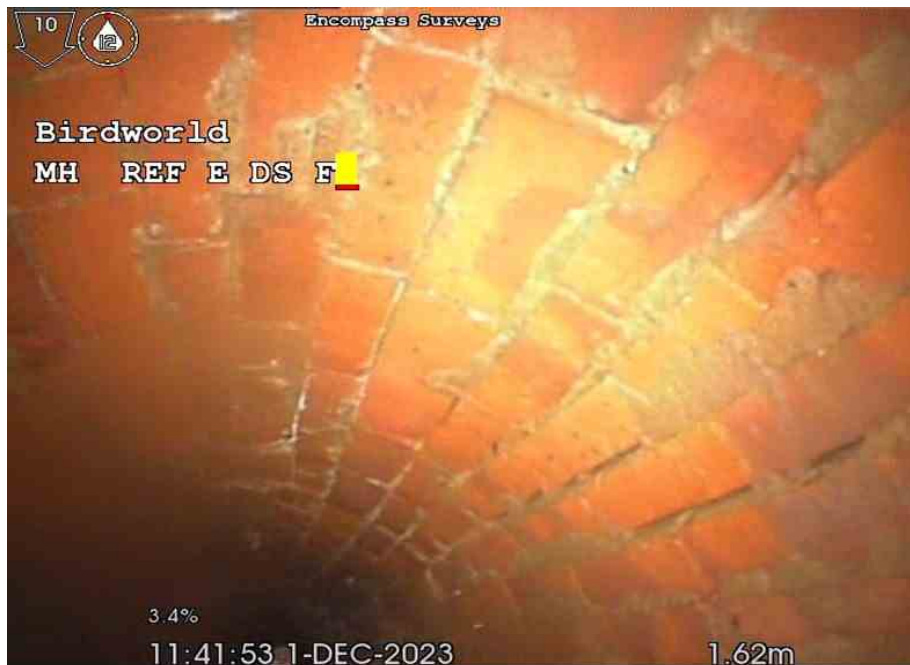
8-1-6A, 00:00:10, 1.62 m Missing mortar, between 5mm and 15mm from 1 o'clock to 3 o'clock
