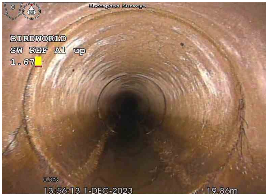
1-1-10A, 00:01:19, 19.86 m Roots, fine at joint
