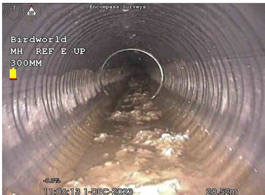
9-1-5A, 00:02:13, 28.52 m Settled deposits, fine, 10% cross-sectional area loss
