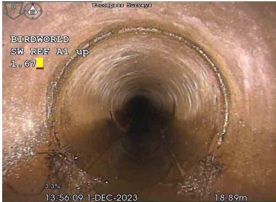
1-1-9A, 00:01:15, 18.89 m Roots, fine at joint
