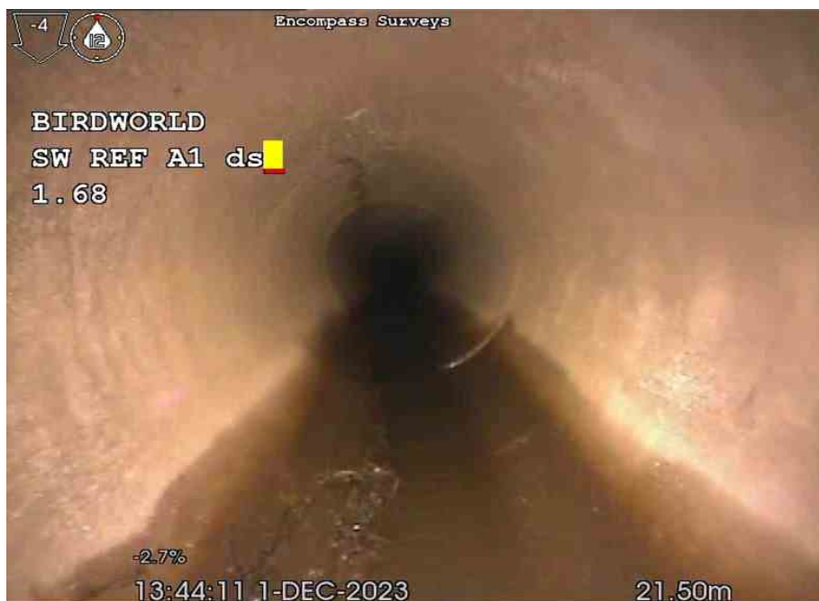
2-1-6A, 00:01:24, 21.50 m Crack, longitudinal at 12 o'clock, finish
