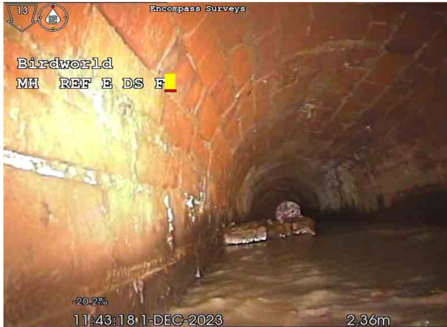
8-1-7A, 00:01:35, 2.36 m Settled deposits, fine, 20% cross-sectional area loss, finish
