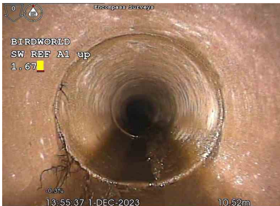
1-1-4A, 00:00:43, 10.52 m Roots, fine at joint
