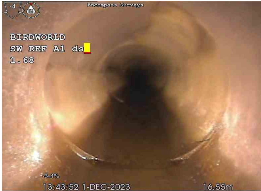
2-1-3A, 00:01:06, 16.55 m Crack, longitudinal at 12 o'clock, start
