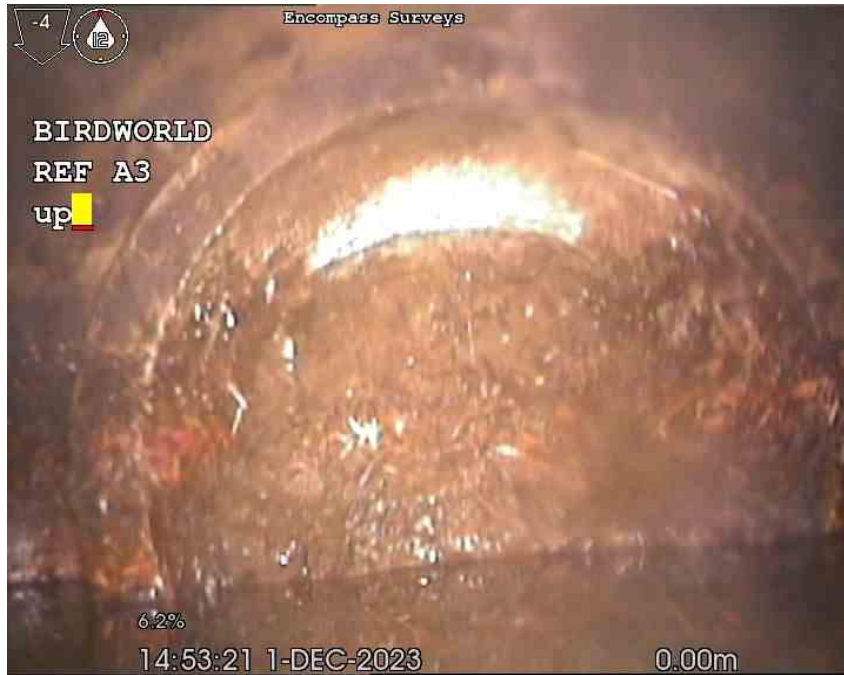
5-1-1A, 0.00 m Start node, manhole, reference: MH (A3)
