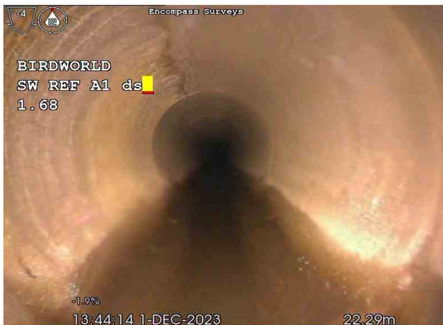
2-1-10A, 00:01:28, 22.29 m Crack, longitudinal at 11 o'clock
