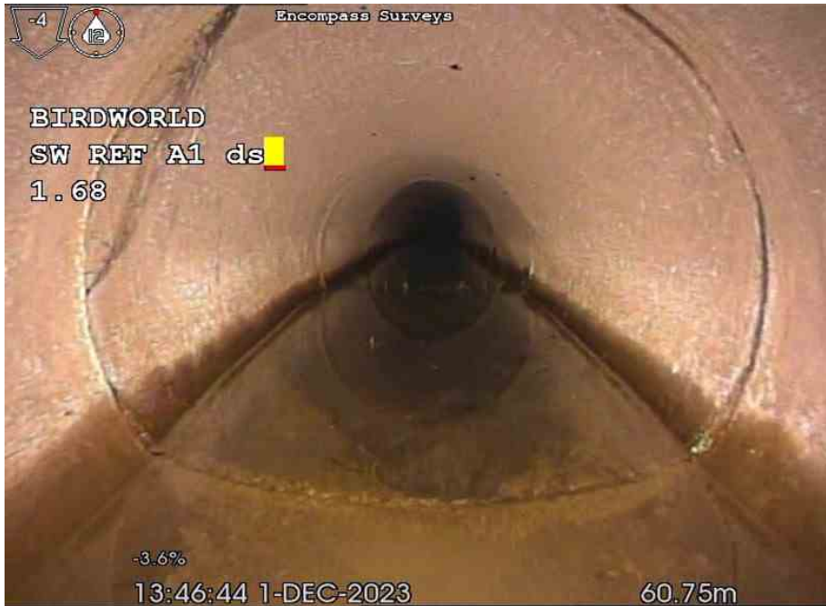
2-1-18A, 00:03:58, 60.78 m Roots, fine at joint
