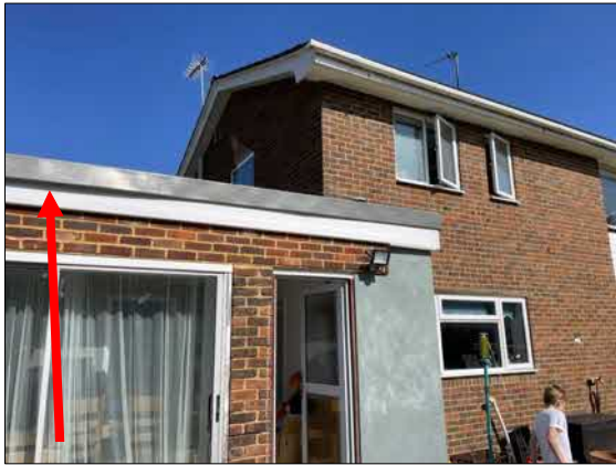
Photograph 3. South-eastern elevation, showing fascia gap
