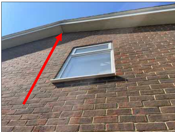
Photograph 5. Northern gable, with apex gap location
