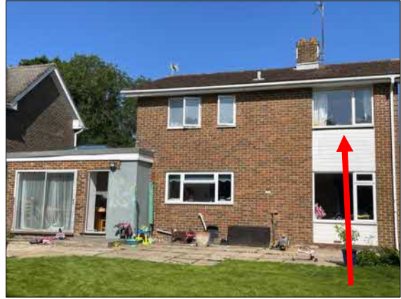
Photograph 2. Eastern elevation, showing gap in cladding
