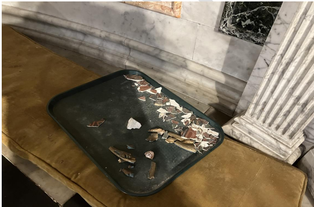
Figure 66 Evidence of progressive loss of painted decoration
