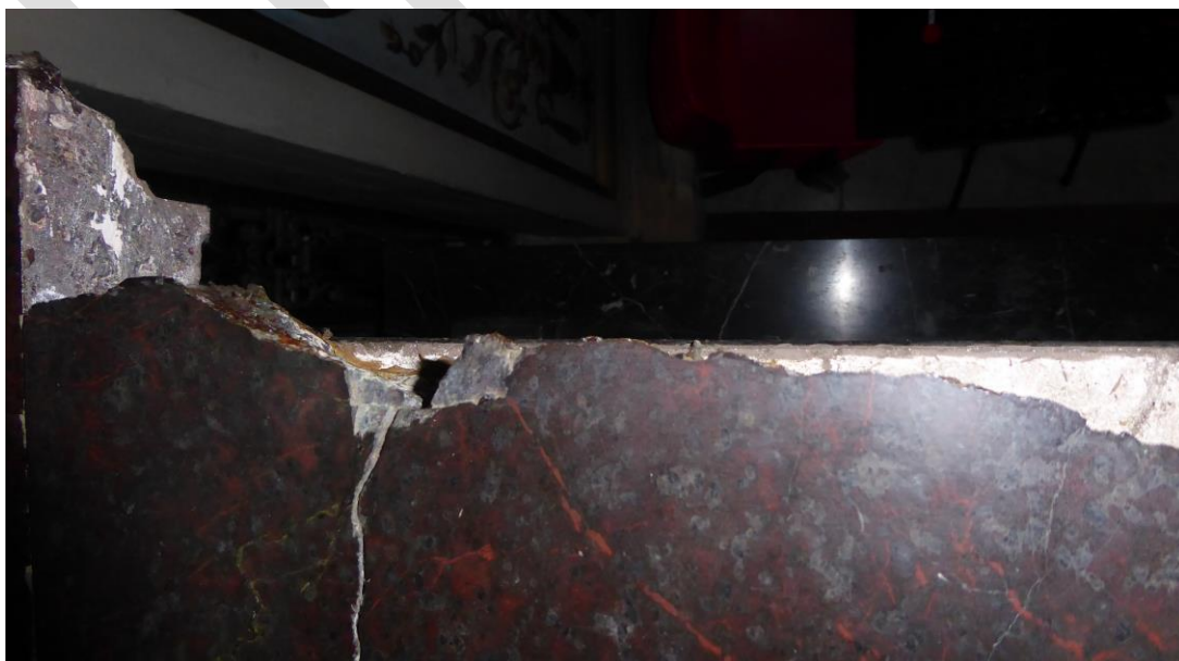
Figure 64 Damage to the marble on the pulpit
