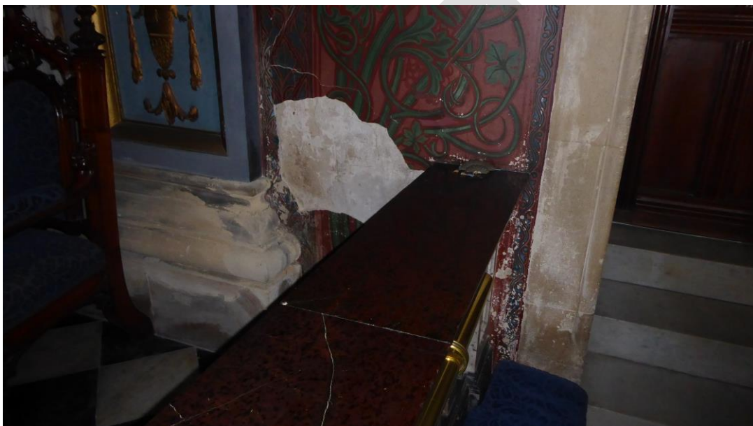
Figure 63 Evidence of moisture ingress damaging the painted plaster
