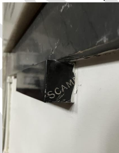
Figure 48 Example of where later dry-lining of aisle wall has partially obscured the signature on the monument
