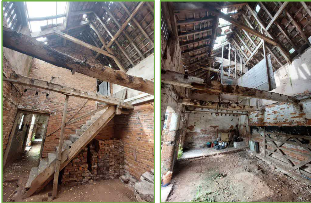
Photo 2 (left) showing large missing section of roof and missing floors. Photo 3 (right) Showing large gaps in the pitched roof and missing floors
