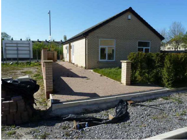
Photograph 8: Building (B1) of modern construction - sealed externally from bat ingress in roof, soffits and verges.
