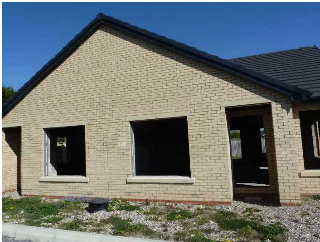
Photograph 9: Building (B2) of modern construction - sealed externally from bat ingress in roof, soffits and verges. Windows and doors not fitted.
