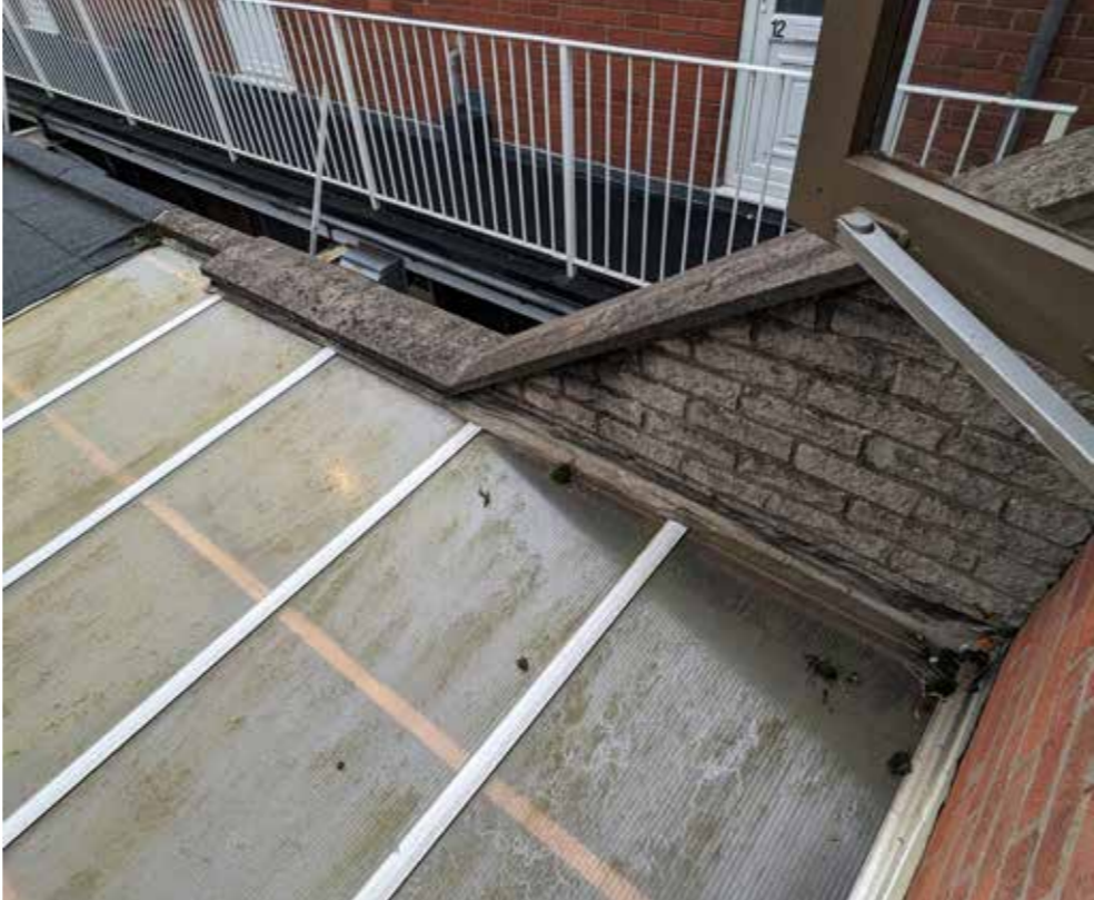
Above: photo taken at first floor level rear window overlooking at existing polycarbonate roof and wall junction, facing south-east
