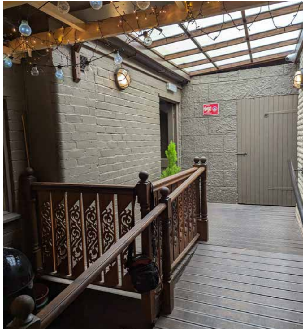
Above: photo taken within ground floor lobby area, facing east illustrating top of existing ramp, balustrade, bin store wall and door and polycarbonate roof.
