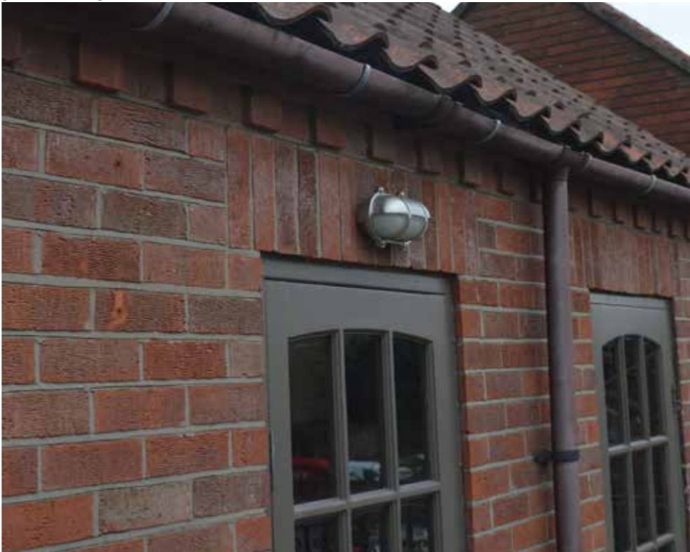
Above: photo taken on first floor terrace area, facing south-east illustrating existing timber framed doors and eaves.
