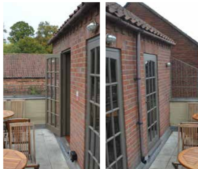
Above: photos taken at first floor external terrace area, illustrating existing timber framed doors.
