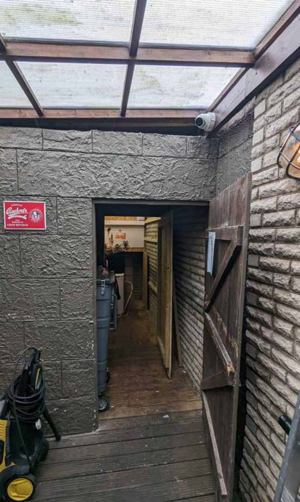
Above: photo taken within entrance lobby area, facing east illustrating polycarbonate roof, bin store timber door and stud wall featuring faux stone plaster to wall.
