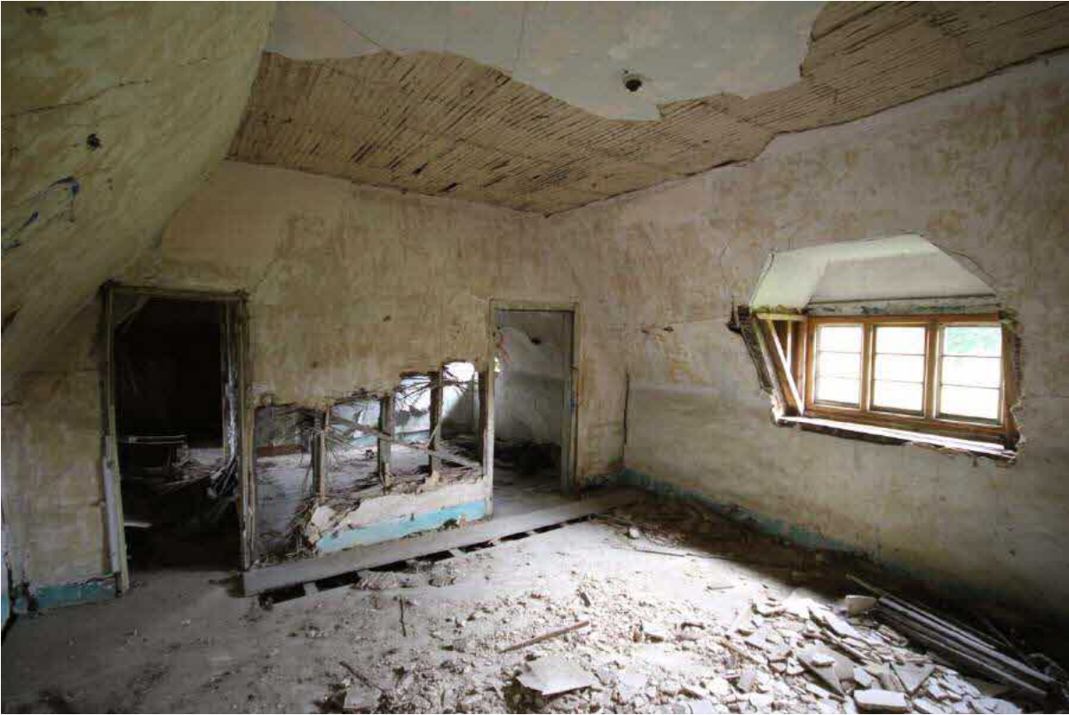
Main bedroom with single board raised for inspection. All boards are to be taken up to facilitate repair and M&E installation.
