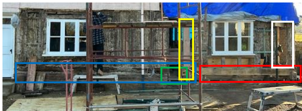
Image 3 showing works to RHS of west elevation. (close up of red box in Image 2)
