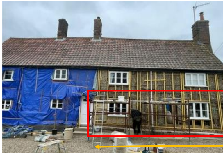
Image 2, West elevation, front door to right hand corner (marked by yellow arrow)
