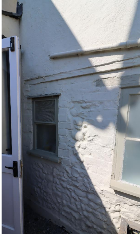
Figure 4: Existing kitchen window to be removed and replaced with traditional timber flush casement window
