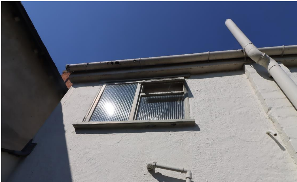
Figure 5: Existing bathroom window to be removed and replaced with traditional timber flush casement window
