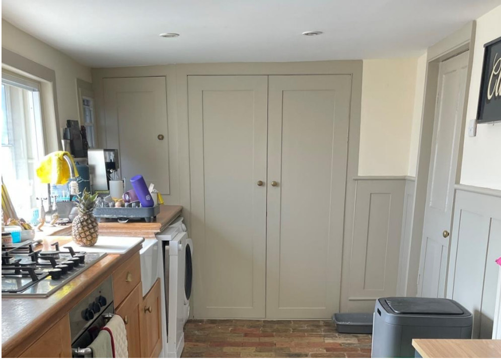
Figure 6: Modern kitchen cupboards to be removed and replaced with partition and door to form new downstairs cloakroom
