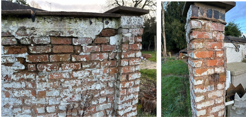
Photo of existing wall – bricks are modern and believed to be from the 1950s
