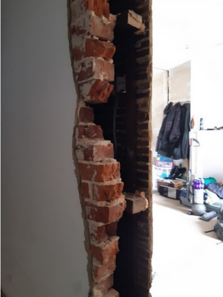
Image 9: Showing the works that were started to create an opening for the new staircase. All works were halted following a visit from the Council.
