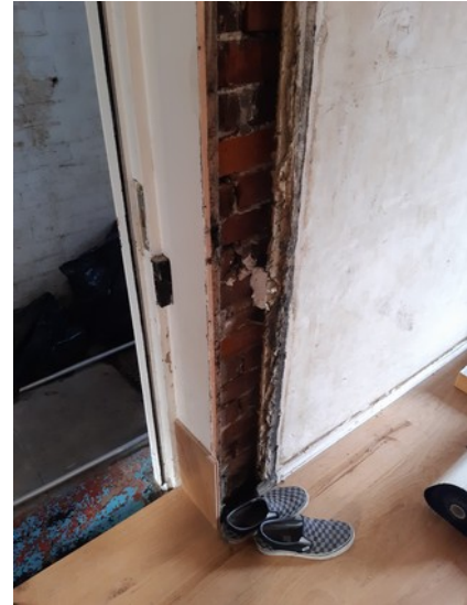
Image 6: Showing the current differences in levels of the floors within the house
