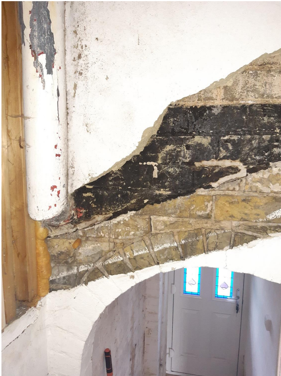
Photograph 5: Detail of the former pitch roof detail over the entrance bay and the rear of the parapet with the later downpipe diverted through the wall above the former roof.
