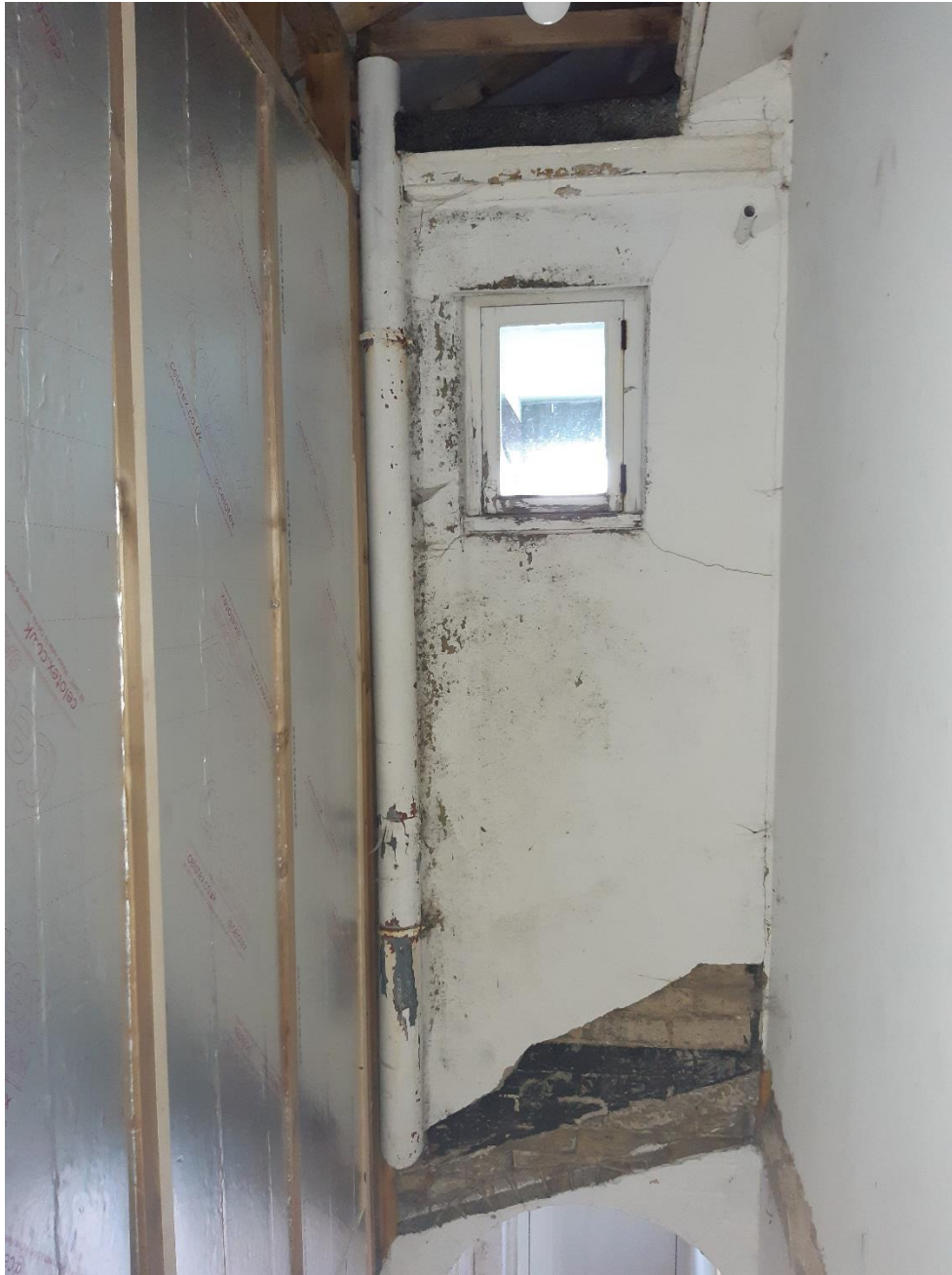
Photograph 4: Interior rear (south) wall of the first floor added storey above the west entrance bay. Note the line of the original single storey roof above the arched entrance and the black bitumen coating to what was the rear of the parapet. The old external downpipe to the added floor is now encased within the building. The foil backed insulation and timber studwork to the left represent the addition or infill between the rear of the front extension and the front of the added wing to the rear of the house.
