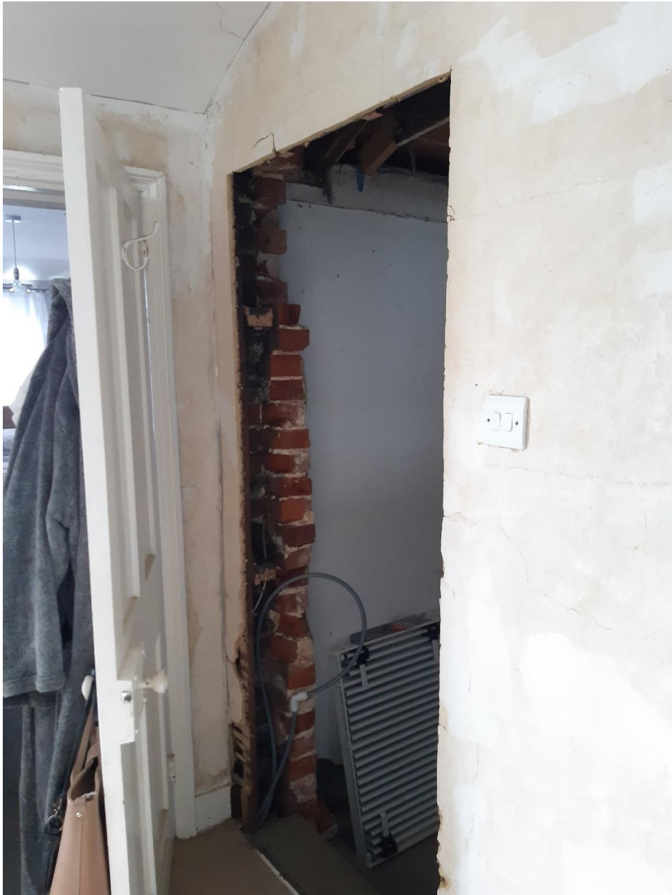
Photograph 10: New opening into the side wall at first floor level providing access from the new stair.
