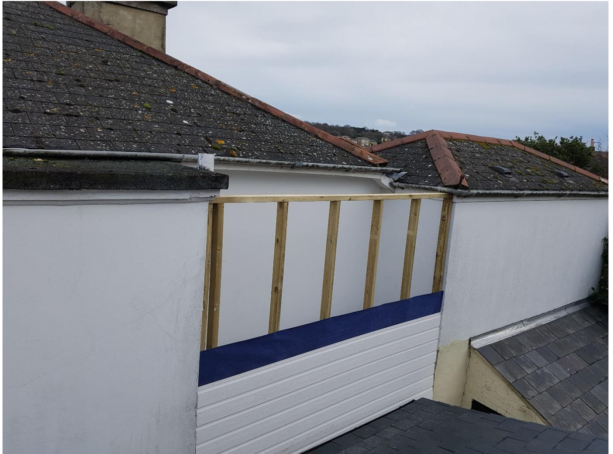
Photograph 8: Studwork of infill extension fitted between the existing eaves of the two extensions either side. External upvc weatherboarding to be replaced with traditional painted timber weatherboarding
