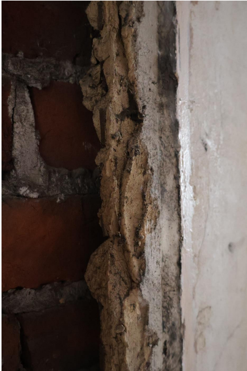
Photograph 12: Detail of internal finish to the ground floor front room, west wall where the door frame had been removed. Note the internal studwork attached to the historic brickwork by lime mortar dabs and the evidence of the traditional 3-layer finish: the base coat of rough plaster with reinforcement pressed into the lathes; the second, thinner scratch coat; and then the very thin, lighter colour finishing coat. The colour and textures of these plasters and mortars contrast with the finish on the first-floor rear room (Photograph 11) and support the suggestion that the first floor rear room has been internally refurbished.
