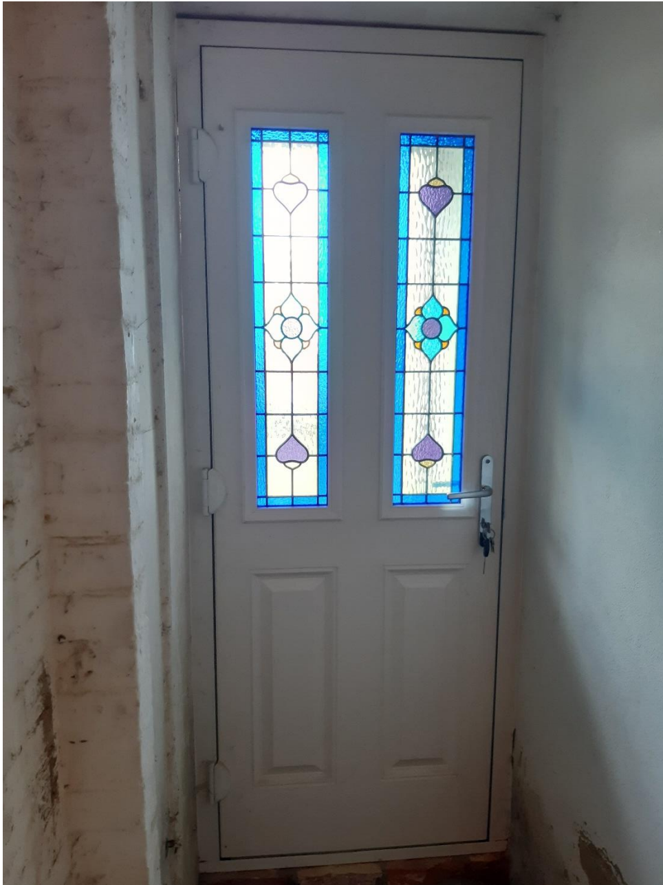
Photograph 3: New composite door and frame to be removed and replaced with timber panelled and part glazed door of traditional design
