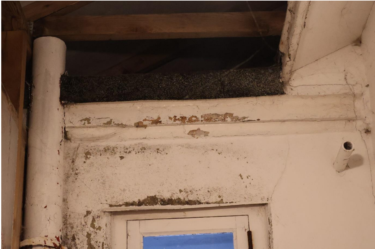
Photograph 6: Detail of the new roof constructed above the flat roof of the former bathroom addition, the earlier eaves of the main house can be seen to the right and the felt edge of the flat roof is to the centre both now enclosed within the new roof.
