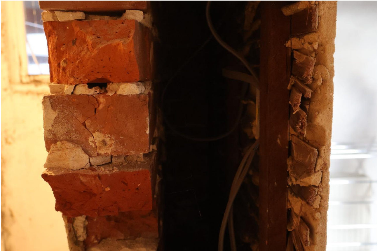
Photograph 11: Section across the newly formed opening at first floor revealing the construction. The red-orange brick with white lime mortar is the historic external wall. To the right is timber studwork of square section with a machine cut finish and sawn lathes. The internal plaster finish is one coat and without hair reinforcement. The mortar is a different mix to that used for the wall and the nature of the construction indicates that it is probably a later 19 th century or early 20 th century refurbishment.
