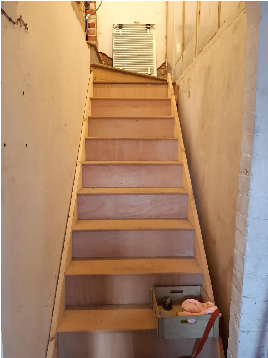
Photograph 9: New stair constructed within the former alley space between the front and rear extensions which has now been enclosed by the infill addition
