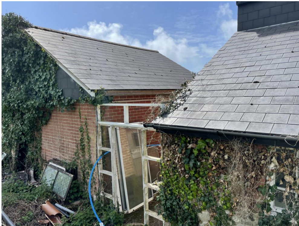
Rear elevation of house and garage showing a link to house with collapsed glazed walkway.
