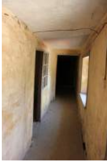
Corridor: note historic plastered walls, lath and plaster ceiling and lime ash or gypsum plaster floor
