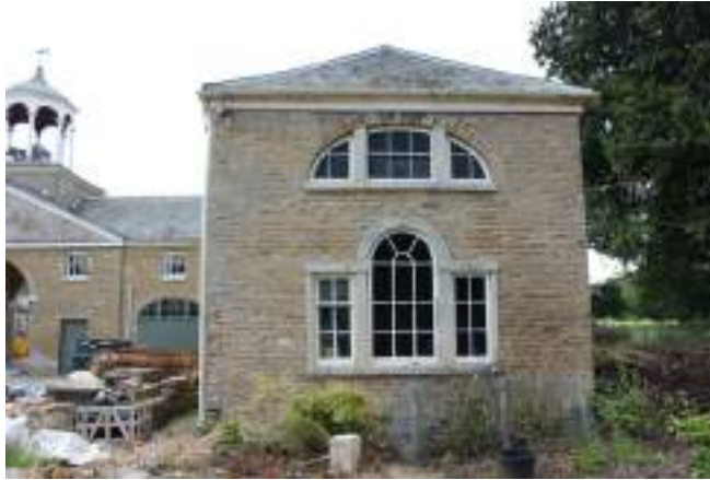
North wing gable end. Both windows, apart from the lower left sash are blind
