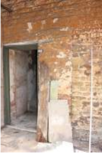
Door to staircase in south wing – note the former opening, now blocked to its right.
