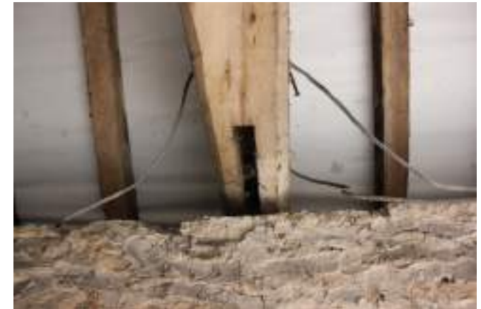
The empty mortice in the north wing hay loft suggest this substantial beam has been relocated and reused
