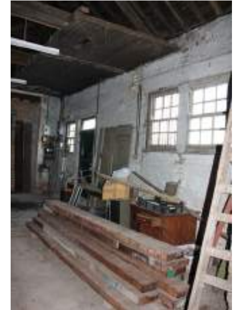
Former boiler house – the gable end double doors on the west elevation are a later modification
