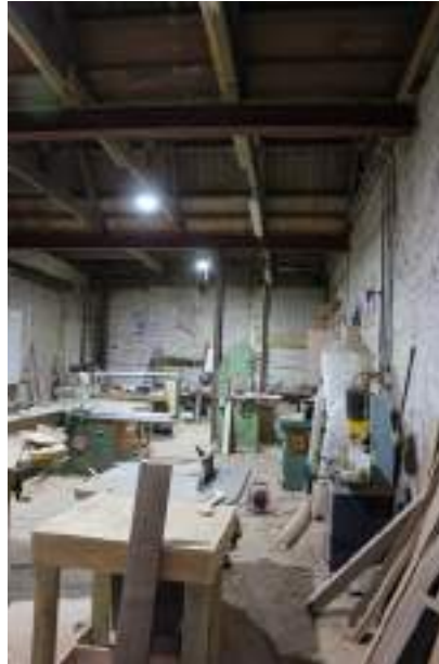
Workshops. This easternmost building abuts the original stable range- note the blocked oculus on the rear wall
