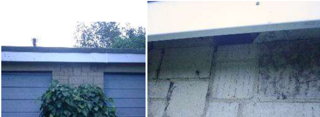
PRF1 – Brick gap in between the garage doors
