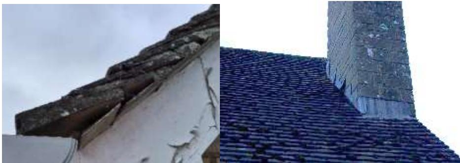
PRF2 – gap in the roof tile mortar (left). PRF3 - gap in the chimney base flashing, second from top (right).
