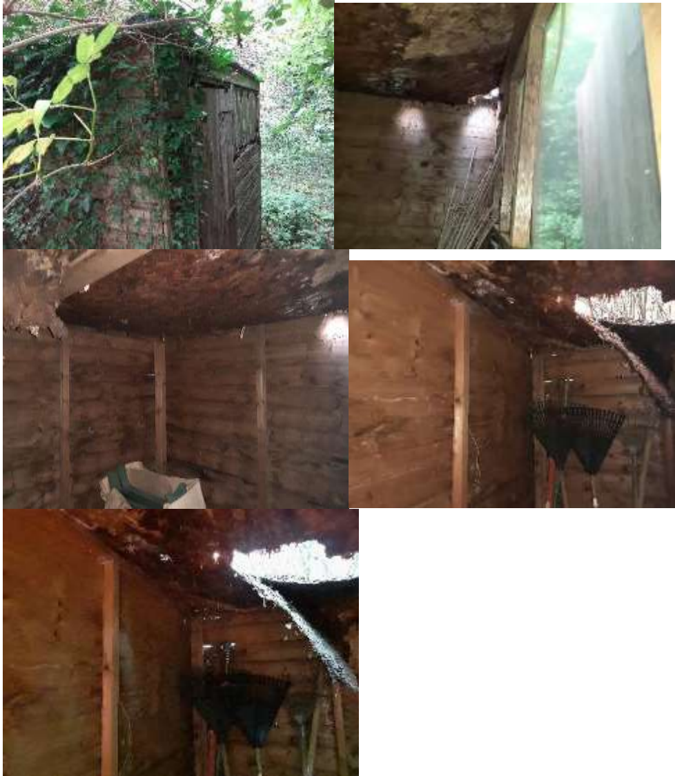
Figure 6: Old shed with holes in the roof (by western boundary), no signs of bats roosting and negligible roost potential due to the holes in the roof.
