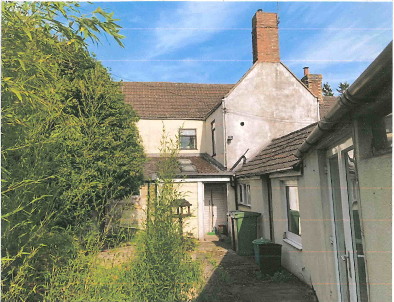
6. View of Cambridge Stores rear facade showing ground floor additions; Note: Proposal to remove additions, re-plan house interior and create new larger walled rear garden
