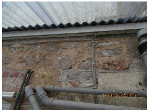
Cement pointing to be replaced
