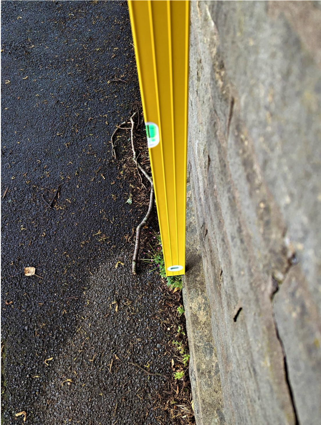
Photograph 02 – Showing the horizontal movement over the height of the retaining wall.
