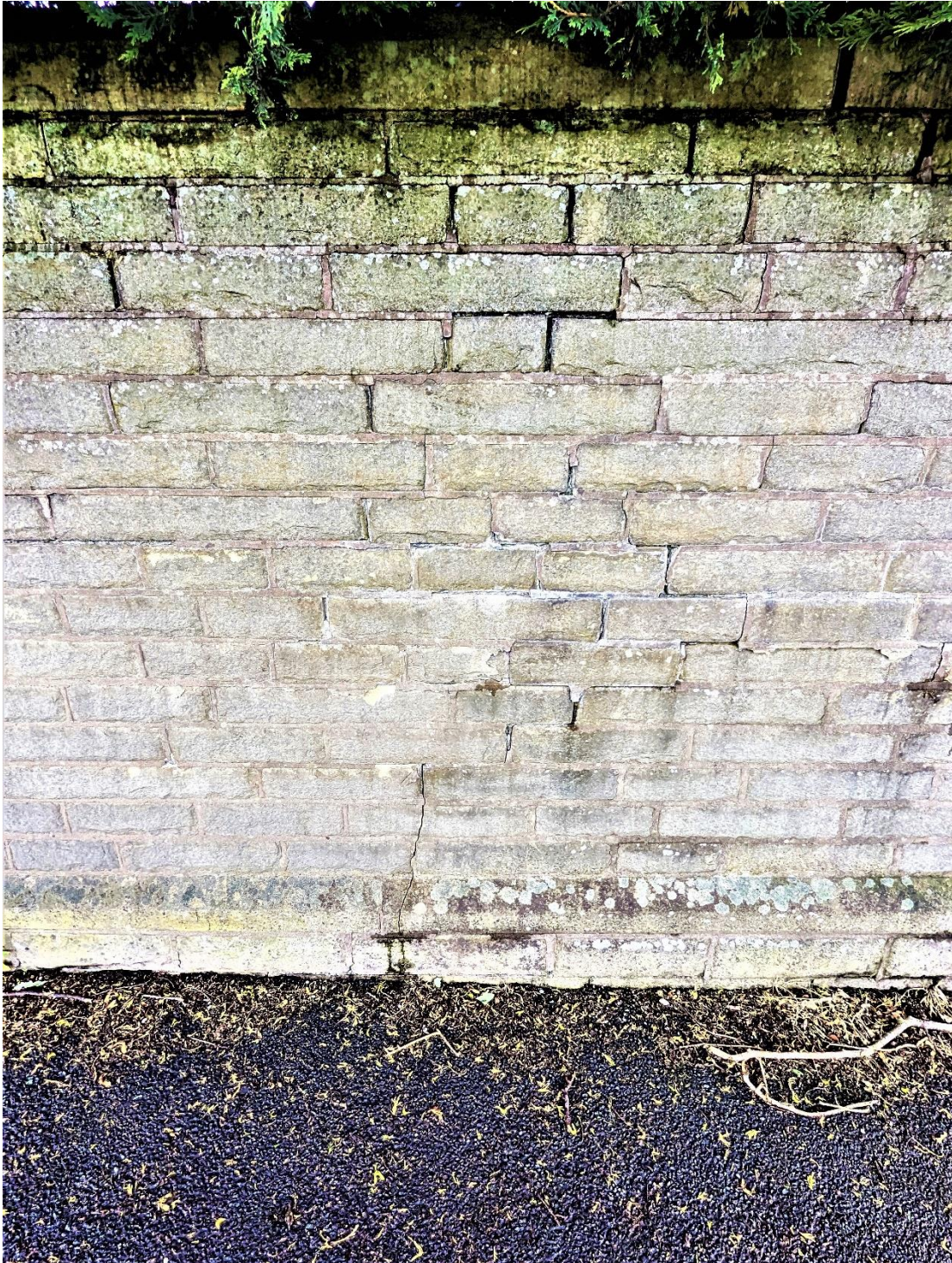
Photograph 03 – Showing a detail elevation of the area most affected by the lateral movement in the retaining wall.
