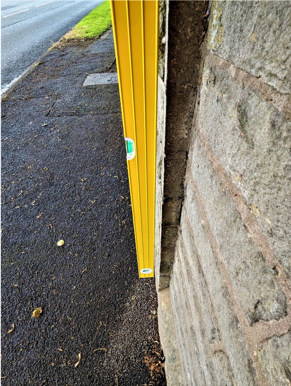
Photograph 05 – Showing the lateral movement at the top of the masonry piers.
