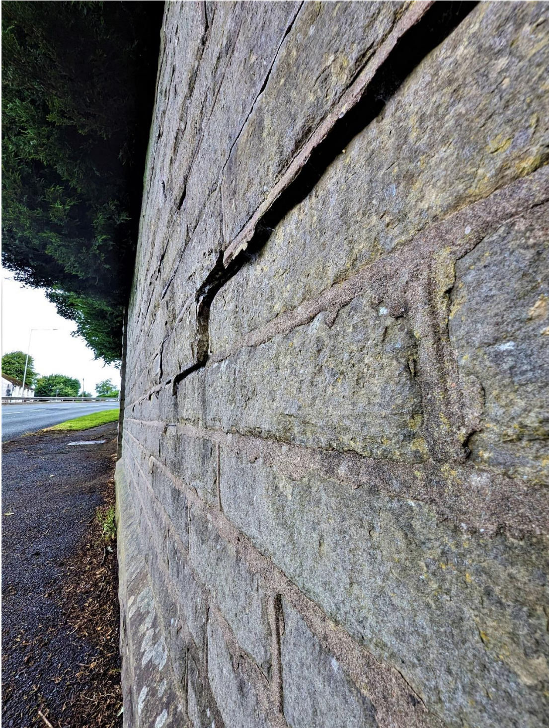
Photograph 04 – Showing the extent of the differential lateral movement of the upper half of the retaining wall.
