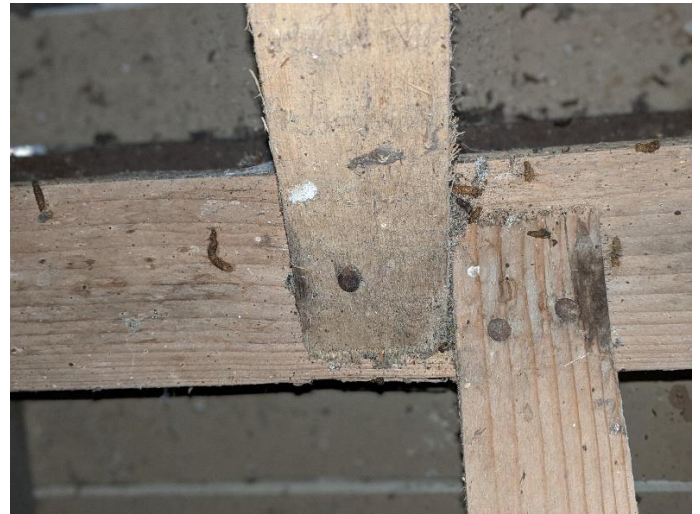
Photo 22 Scattered BLE droppings on a beam in the attic of barn
