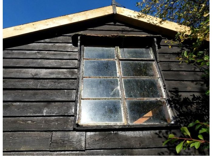
Photo 20 Warped timber cladding on the south gable end of the barn.
