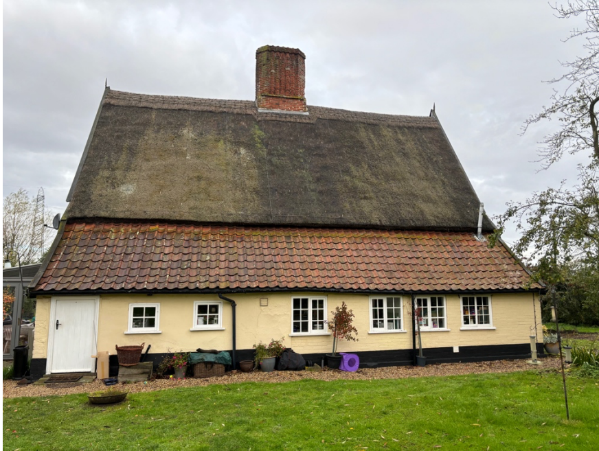
East Elevation of Perkins Farm showing much altered northern section of lean-to.
