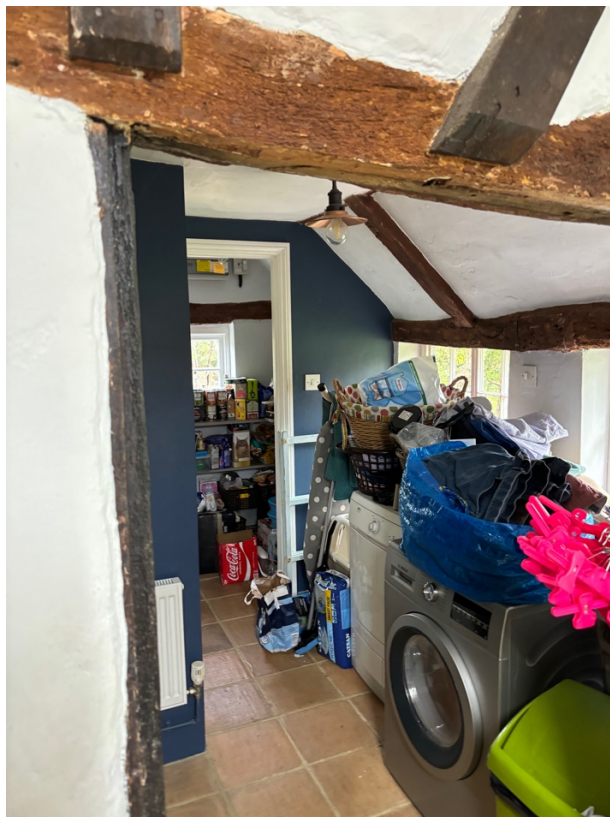
Internal photo showing C20 partitions (painted blue) proposed for removal (with contemporary frames, architraves and door)
