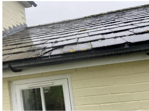
Broken tiles and minor lifted tiles on the eastern single-storey wing of the house. (looking northeast)
