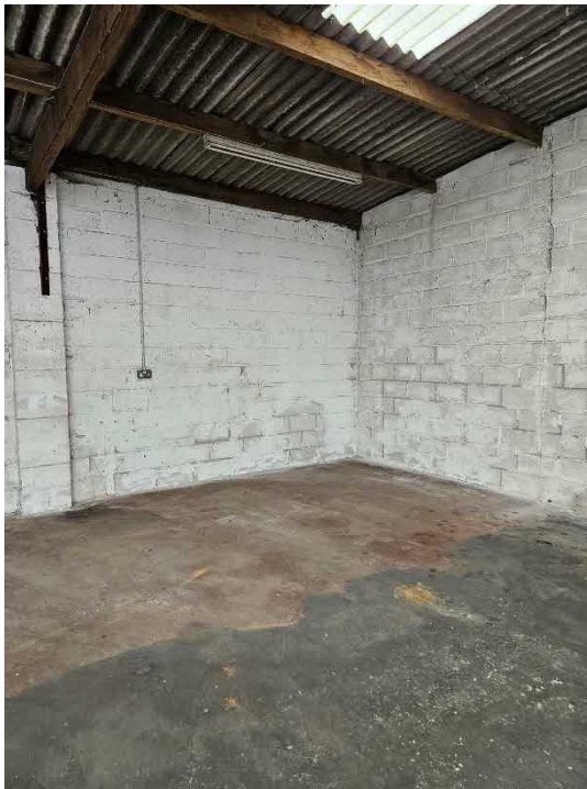
Figure 2: The internals of room 1 on the northern end of the building (top left), room 2 (top right) and room 3 to the south of the building (bottom left).
