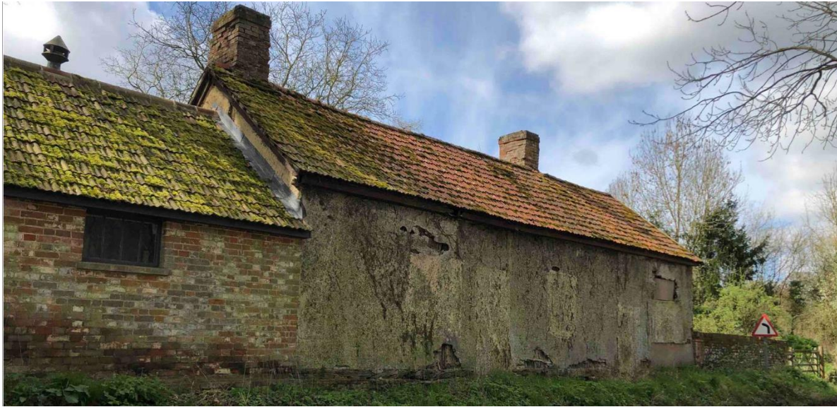
North elevation showing poor state of render, evidence of existing opening, some partially infilled and 2 chimneys evidence of 2 cottages
