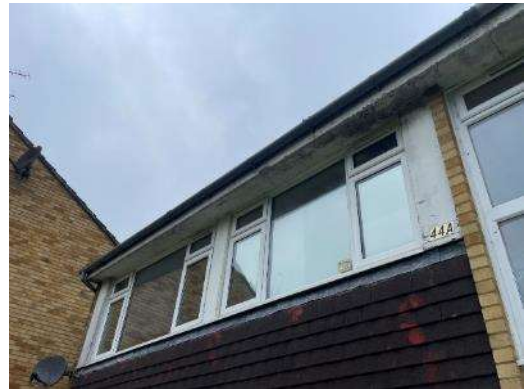
Fig 09 – Fascia & soffit condition.
