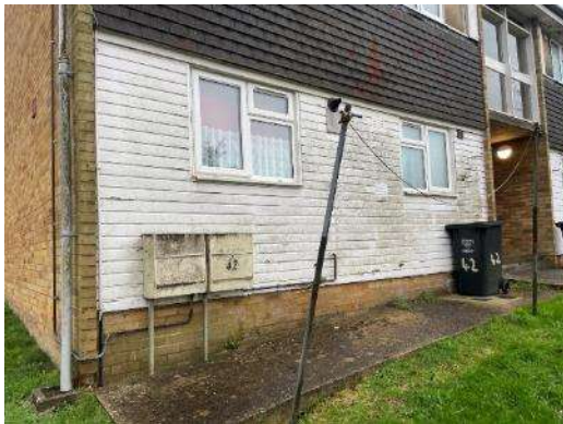
Fig 12 – Rear gas meter box condition.
