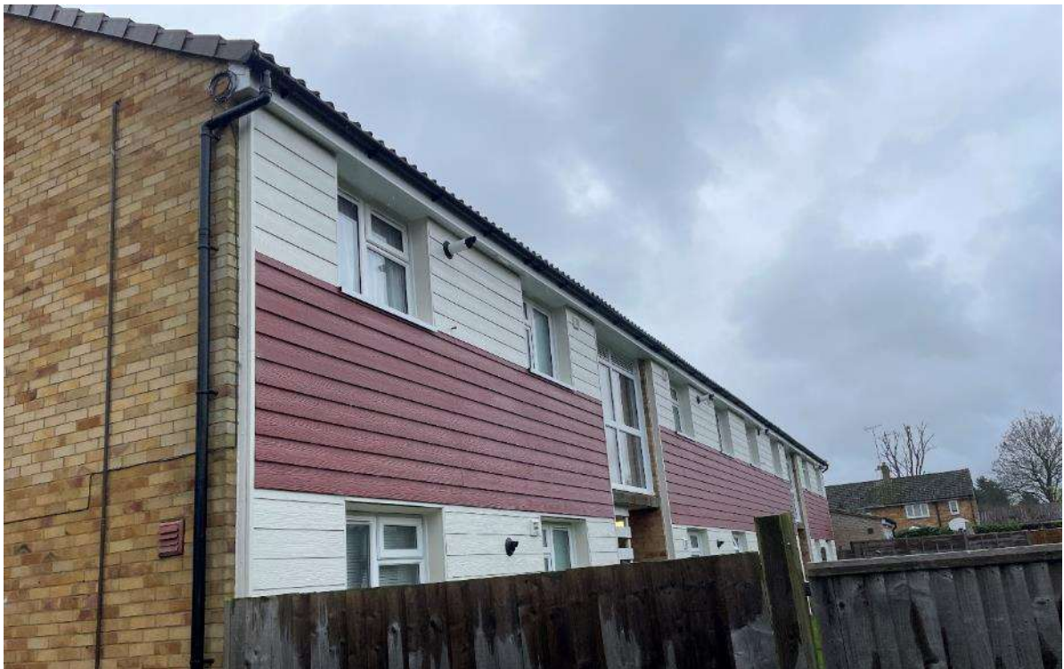
Fig 18 – Close up view of refurbished rear elevation of Block 6-9A Sebright Road.
