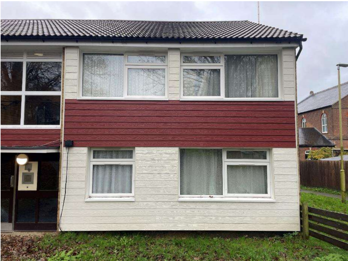
Fig 16 – Part close up view of refurbished front elevation of Block 6-9A Sebright Road.
