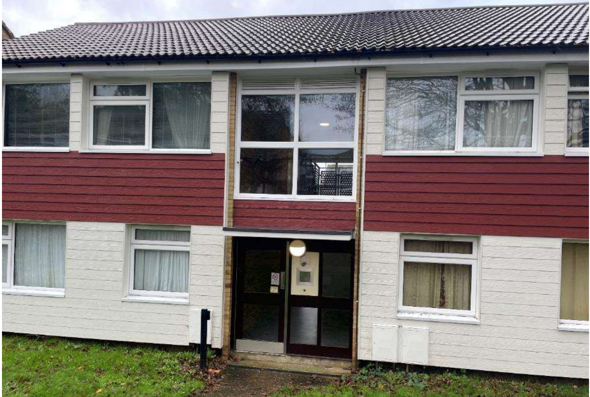
Fig 17 – Close up view of entrance canopy & recessed gas meter boxes of Block 6-9A Sebright Road.
