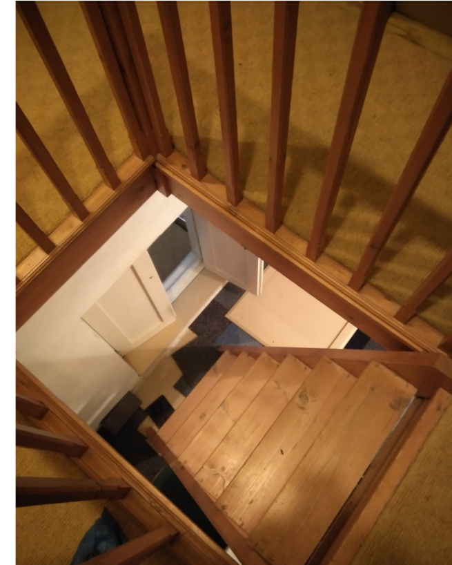
figure 2.2 compromised access to the loft
