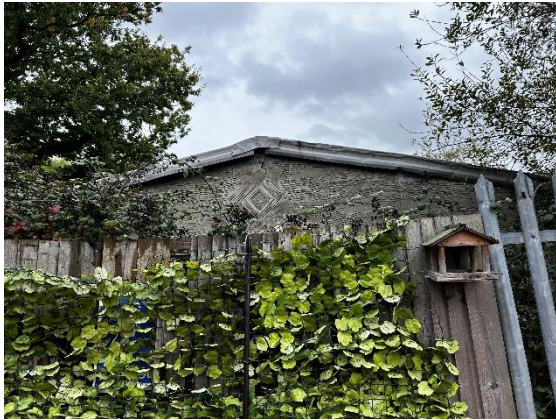
Photo 1 – Crevices under fascia of Building B4
