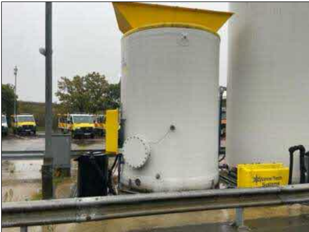
Salt saturator tanks
