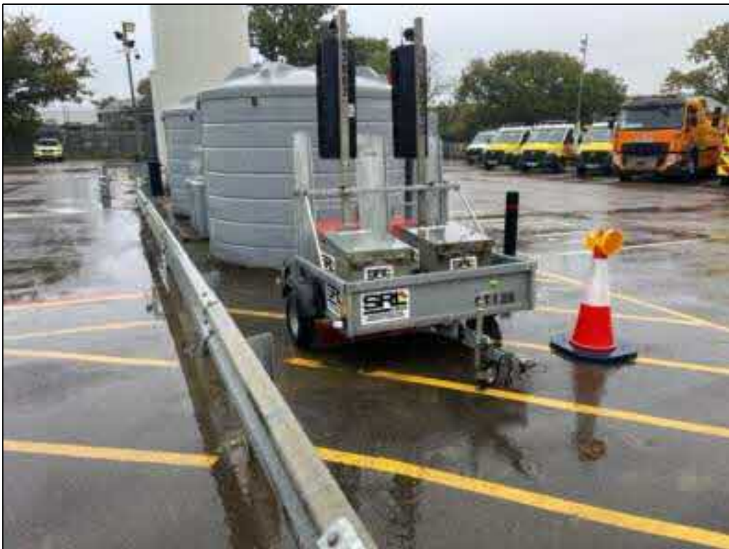
Above ground fuel tanks
