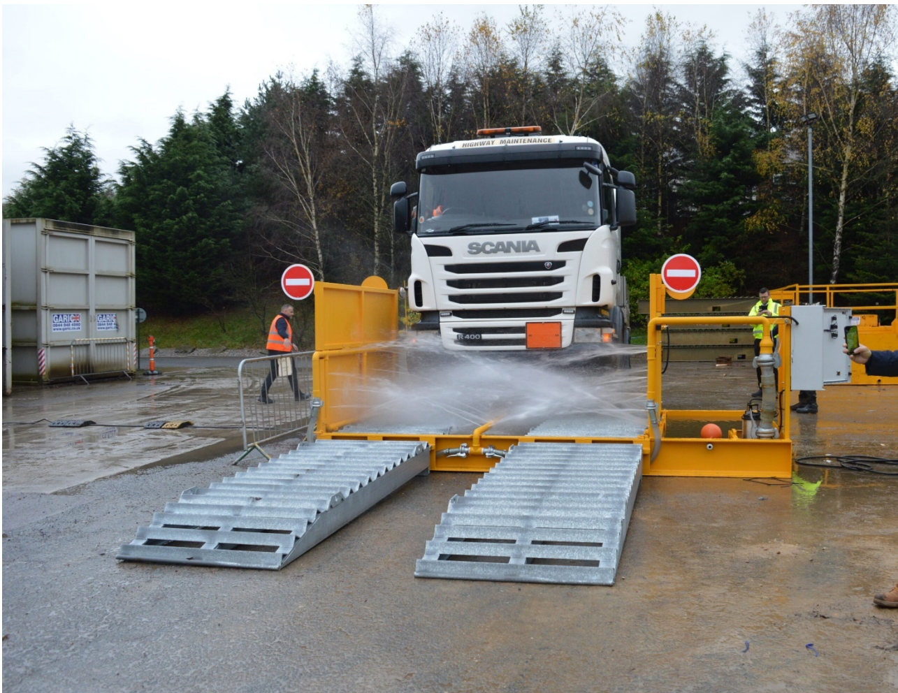
Figure 7: Wheel Wash Facilities prior to HGV vehicle exit
