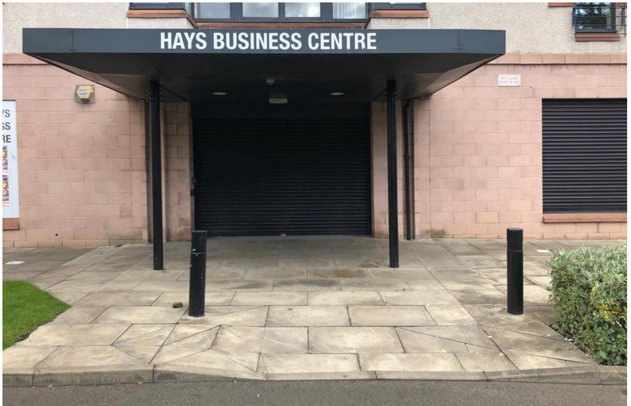
Photograph of existing external level surface treatment to entrance [level access will be maintained for the new entrance design]
