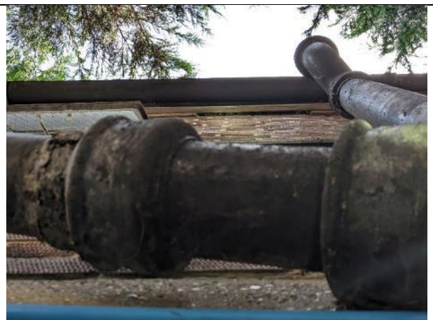
Photograph 14: Gaps beneath fascia on Building 5
