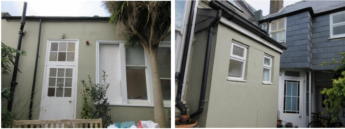
Figure 6 (left): Side (east) elevation of the rear extension to no. 26A, which addresses the garden of the Site.
