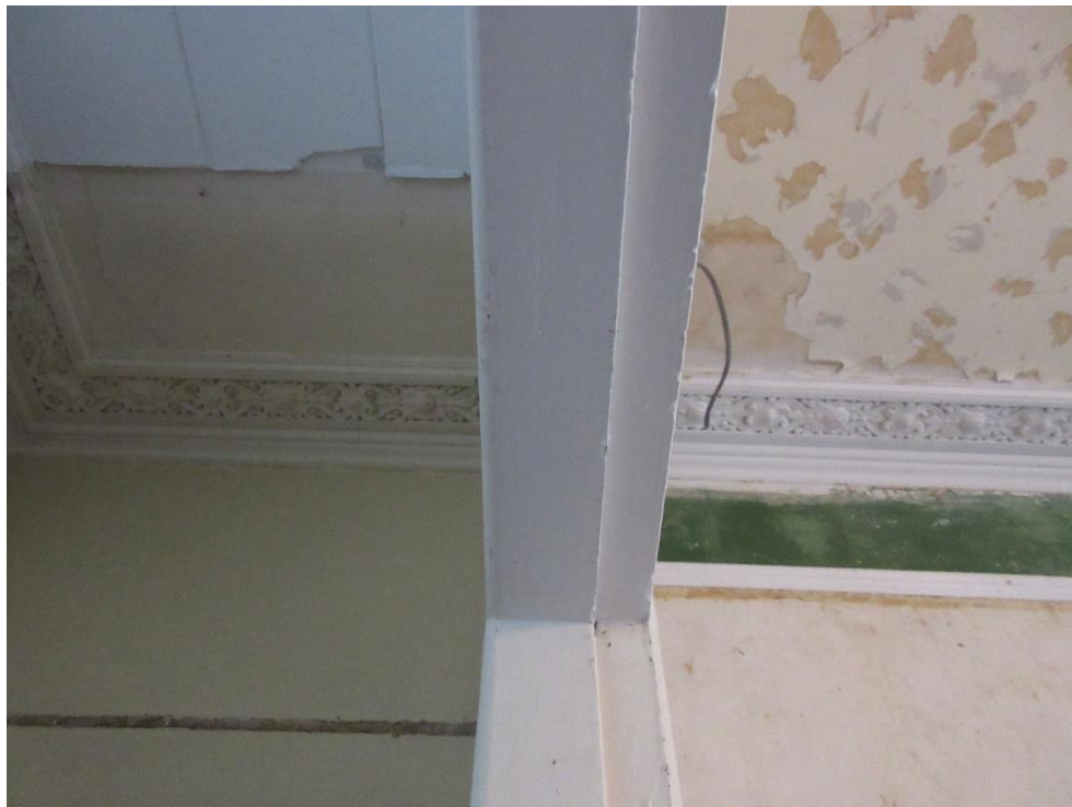
Figure 14: Ground floor – Drawing room. Note original cornicing and picture railing, and modern stud walling.
