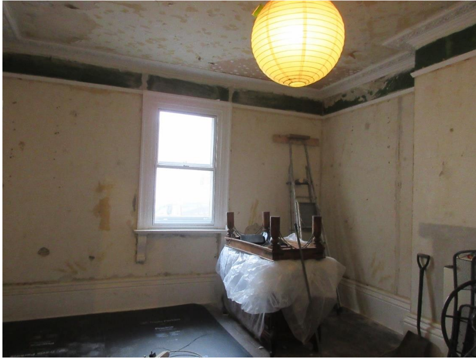
Figure 13: Ground floor – Drawing room. Note original window surround, brackets beneath window cill, skirting, cornicing and picture railing, and chimney breast.
