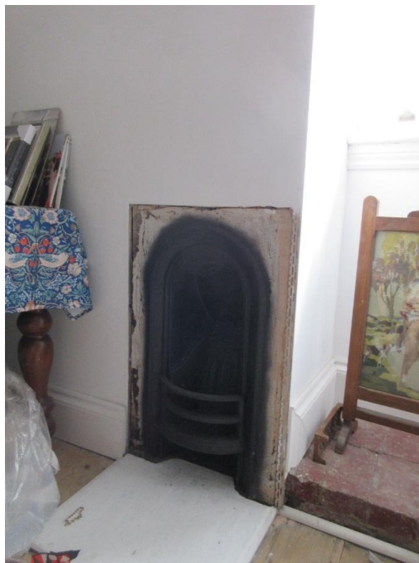
Figure 22: Attic floor – South room. Note historic fireplace located immediately adjacent to modern “alcove” with modern window.
