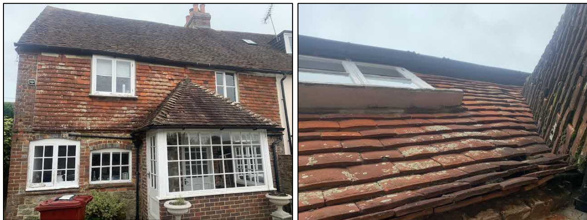
Photographs 1 & 2. The western face of the property and evidence of tile gaps visible at the property consistent with descriptions from the bat scoping report by AEWC.
