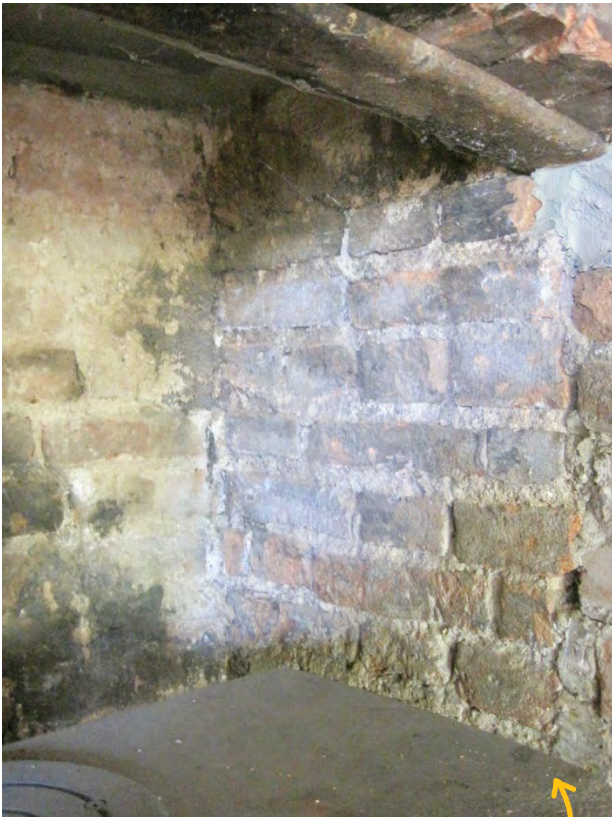
Bottom Left: the side walls and fire-back in the chimneybreast at Stirrups. These are Tudor era bricks.
