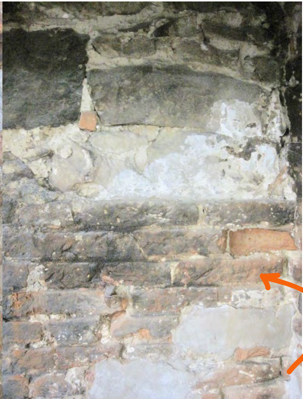
Above, Right: the 2-inch hand-made bricks in Living Room chimneybreast at 330 Grove Street Petworth.
