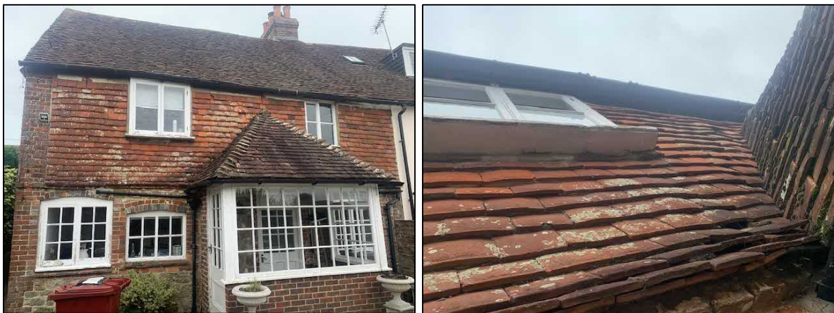
Photographs 1 & 2. The western face of the property and evidence of tile gaps visible at the property consistent with descriptions from the bat scoping report by AEWC.
