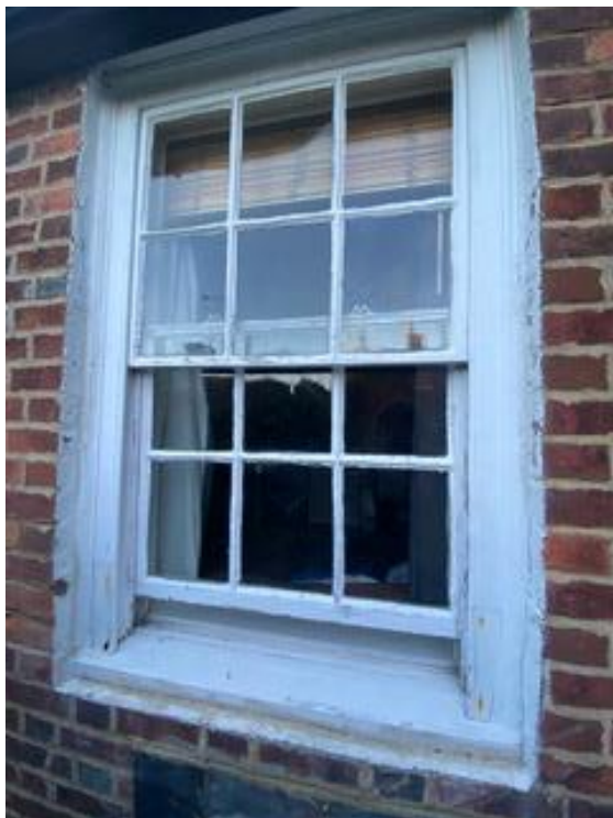
Photo C – closer view of W3
